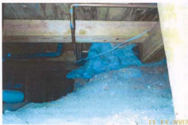
Fig. 95 2002 photo by Nancy Niedernhofer of plumbing system installed in 1997. Plumbing should be monitored annually for leaks due to severe weather to prevent moisture damage in foundation and subflooring. View facing E
