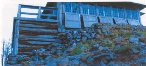
Fig. 61 The west wing foundation is in good condition. Note some deterioration to rock pile. Maintain rocks annually as they shift and reduce support of west wing foundation. Facing E
