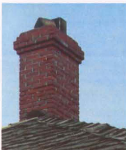
Fig. 72 Note deterioration on lower mortar joints. View facing NE
