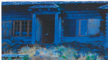
Fig. 84 8-lite casement windows on central hall. Note evidence of moisture trapping at sill level from shutter. View facing N
