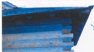
Fig. 77 Exposed rafter tails experience highest deterioration of roof framing. View facing W
