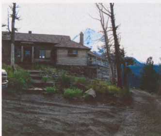
Fig. 52 Cloud Cap site at entrance. Note vehicle induced erosion and deterioration of stone barriers along road and path. Facing S
