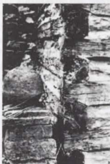
Daubing composed entirely of portland cement is never appropriate to use on a historic log building. Photo: NPS files.
