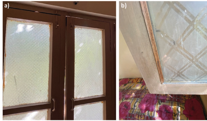
Figure 2.9. Windows in a contemporary structure showing: a) visible gaps between window sash and frame, and b) missing glazing stops (photographed by author Y.I., 2021).
