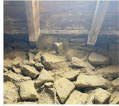
c) Hybrid plastered wall: Mud plaster removed, exposing stone structure and mud mortar.
