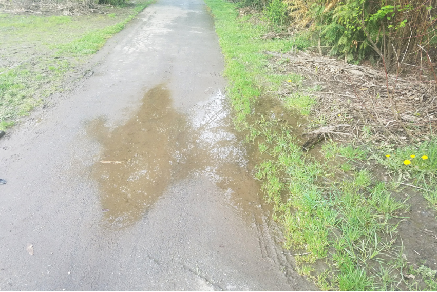
Figure 4: Surface impermeability causes standing water to accumulate
