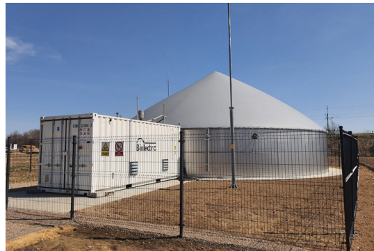
A biodigester converts sludge to methane and “digestate,” an organic fertilizer. Source: PigProgress.net
