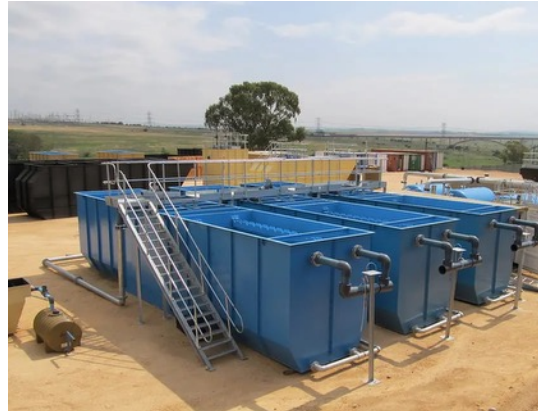
A packet waste water treatment facility in South Africa. Source: WEC Water
