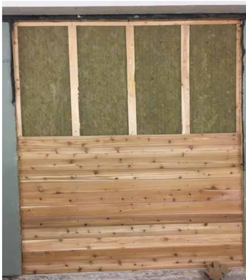
Figure 5: Specimen with membrane, insulation, and partial cedar siding
