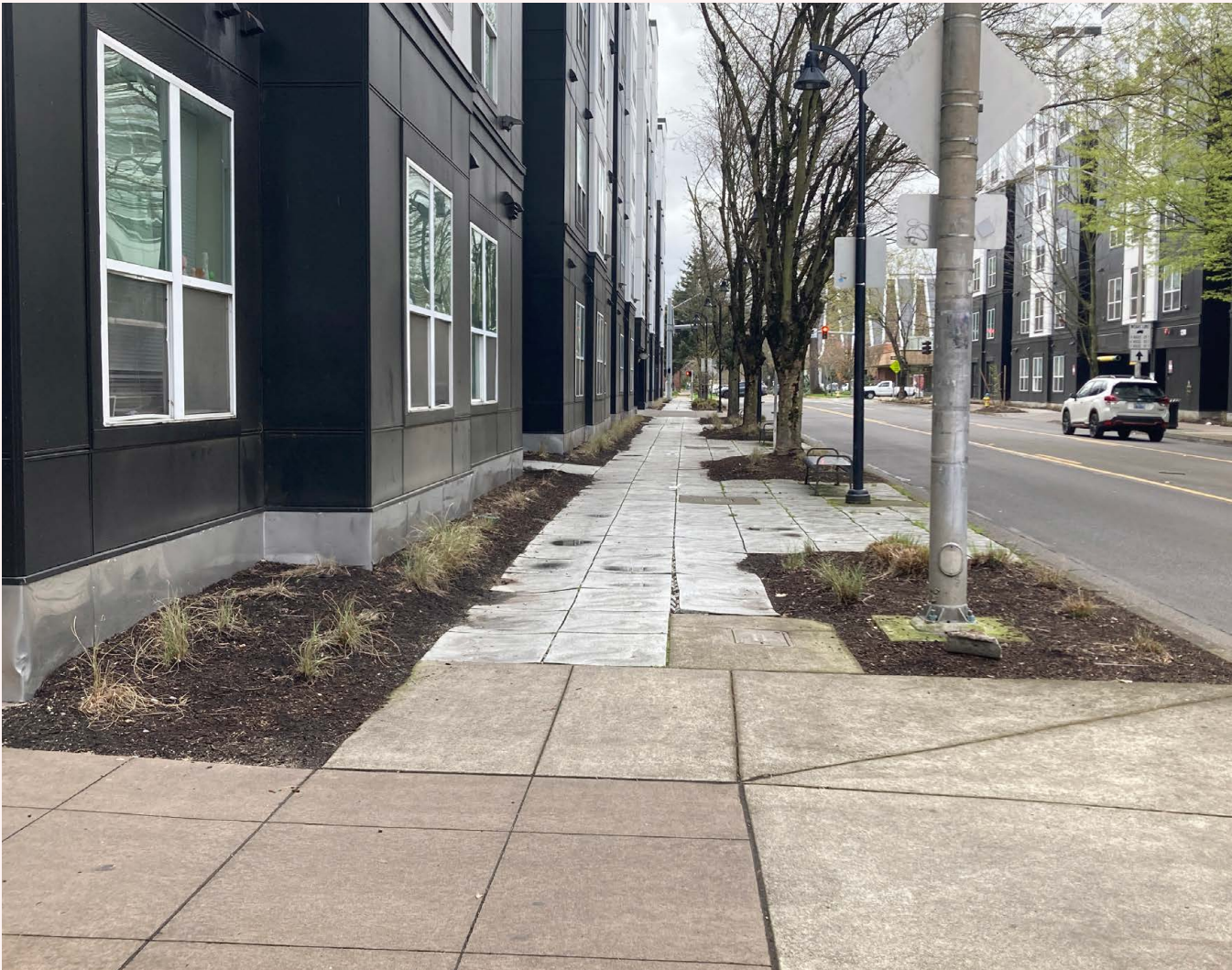
Figure 1.3.15 Terrewalk System Failure
