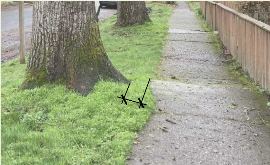
Figure 2.4.28 Visualizing Root to Sidewalk Distance Annotated field photo illustrating the distance between visible roots and the adjacent sidewalk.
