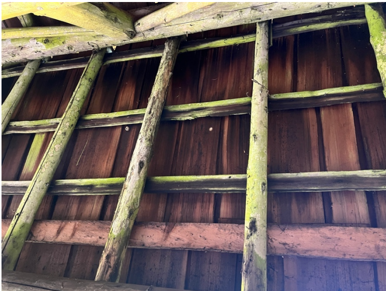
< Example of deterioration of purlins and rafters; note previous purlin replacement
