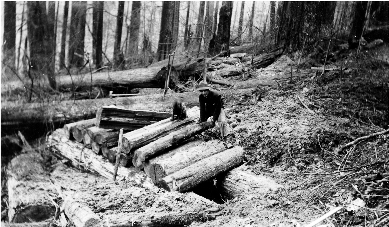
Caption of the photo reads: Olympic N.F. Building a Wooden Trail Culvert c. 1905.
