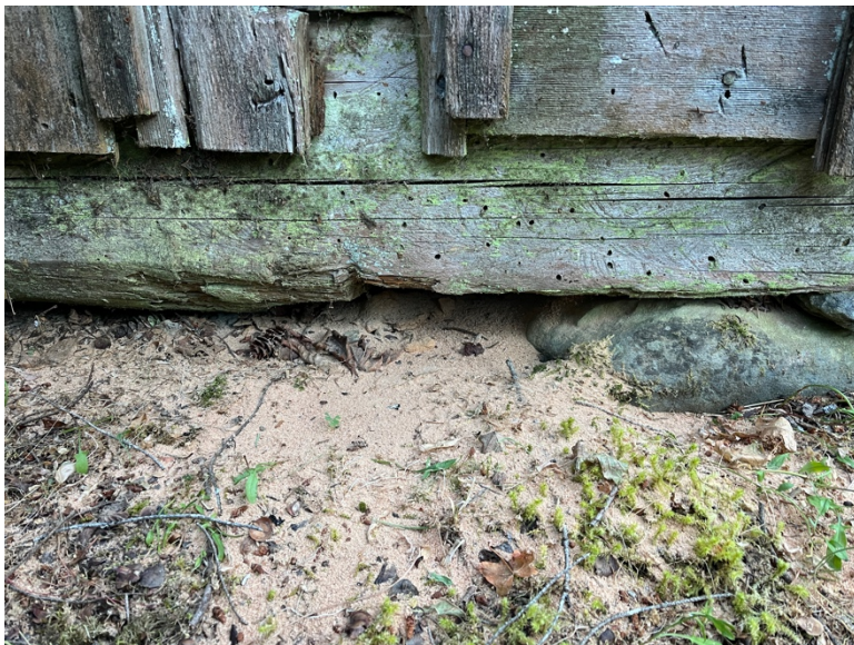
< Evidence of powder post beetle deterioration on west elevation sill log
