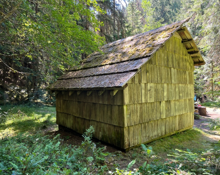
< North and west elevations showing debris and bio-growth on roof shakes
