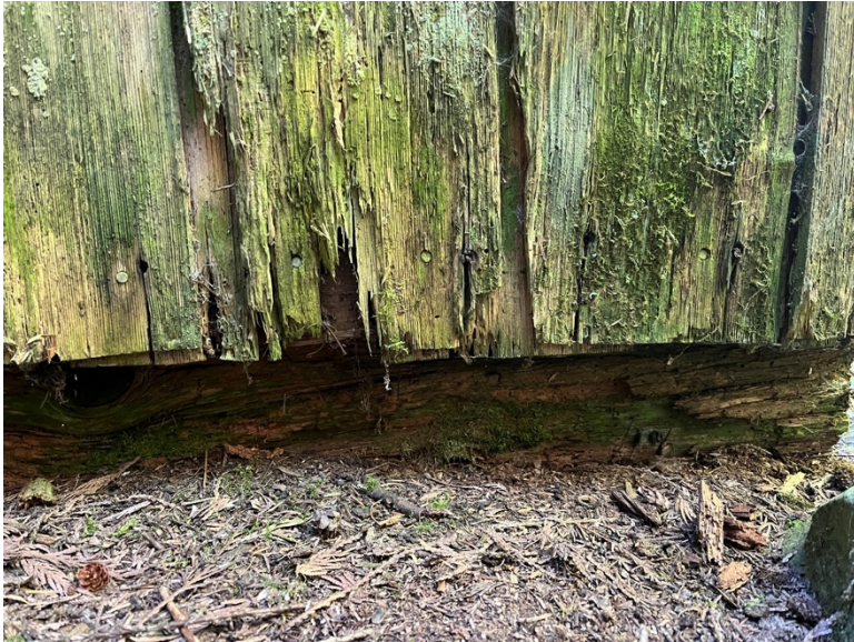
< Example of shake deterioration present along bottom course of north elevation; note deterioration of sill log at ground contact
