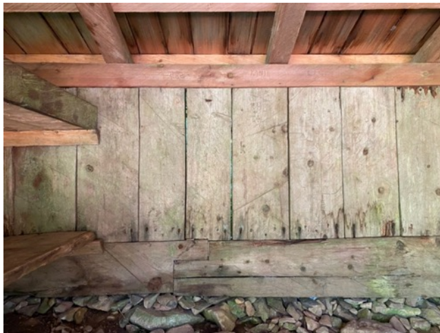
Note: sill long joint repair and eras of wood quality evidenced by differing color
