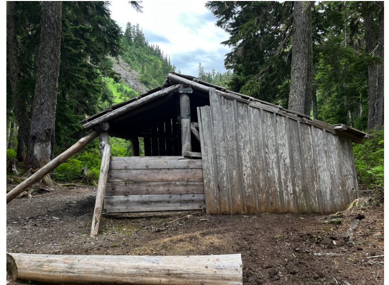
^ East elevations showing diagonal logs added to stabilize structure; missing east elevation siding boards replaced with horizontal boards
