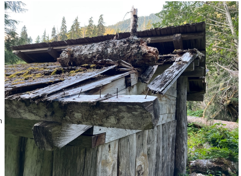
Detail of damage on NW corner of roof structure >
