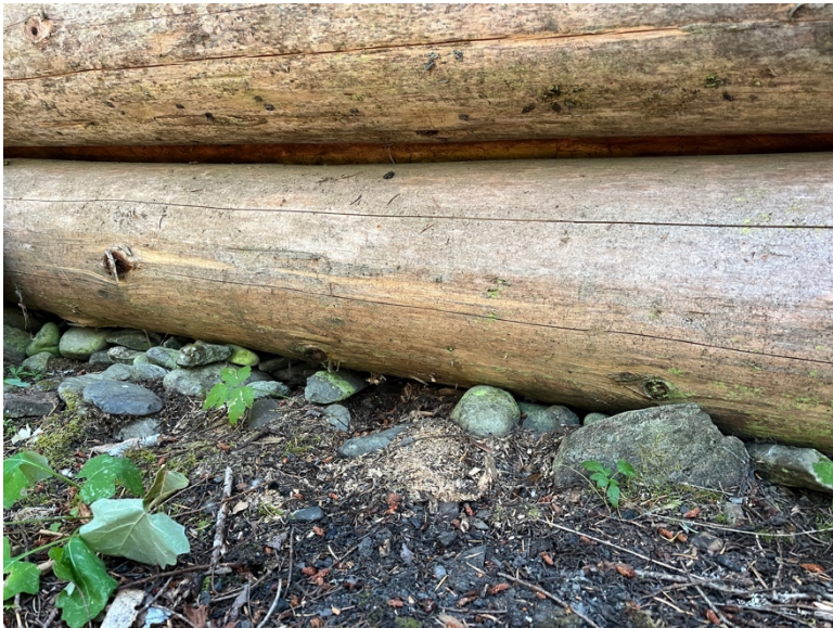
< Potential evidence of critter burrowing between foundation stones
