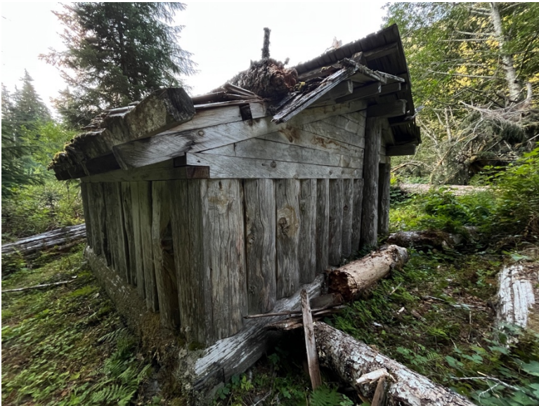
< North and west elevation showing tree damage to NW corner roof structure
