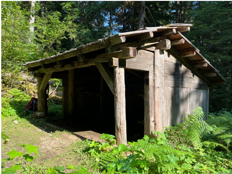
< West and south elevation showing vegetation encroachment
