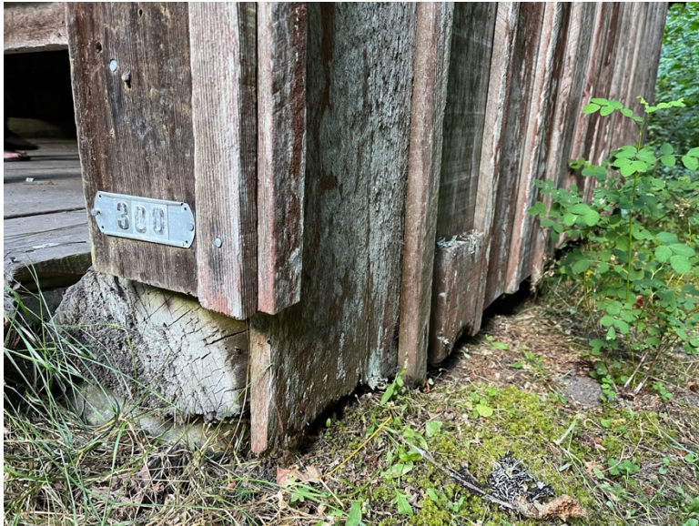
< Detail of mild water damage along east elevation siding boards; red bio growth throughout; organic growth on sill log
