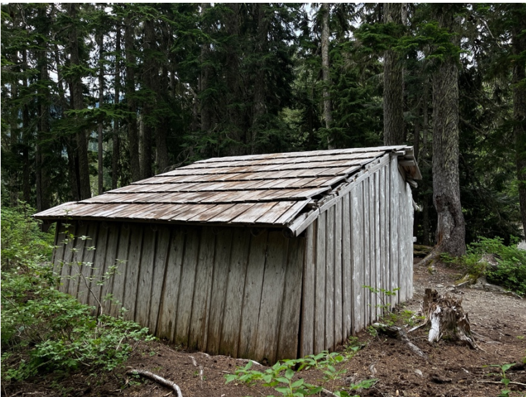
< North and west elevations showing ground contact deterioration on siding boards; roof and siding shifted due to structural lean toward east; exposed rafter missing shakes on western edge
