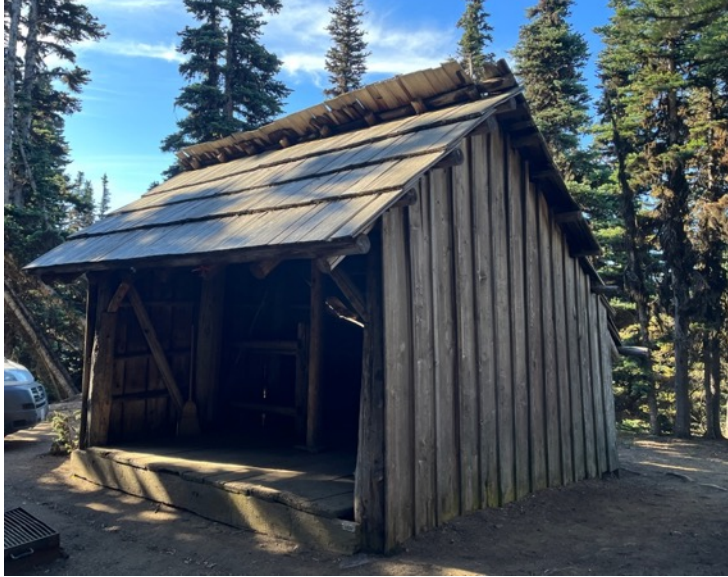
Left: Deer Park 1 shelter is one of two identical shelters built in 1930 of the USFS construction design. The original shake siding was replaced with board and batten in the 1950s. Photo by author.
