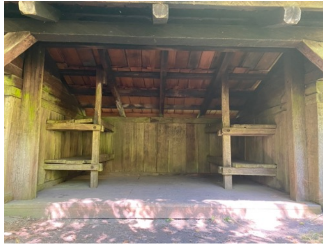
Note: used of plank flooring and blackening of roof beam due to proximity of unofficial firepit
