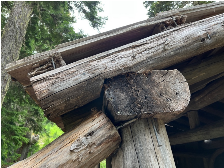
< Example of deterioration present on many of structural roof members
