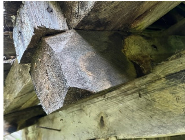
Note: chamfering detail found of majority of roof members on shelters of Mission 66 era
