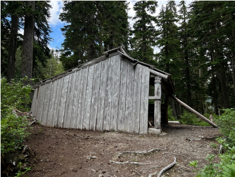
< West elevation showing missing board and batten siding; damaged purlin end; mild ground contact deterioration on siding boards; missing upper trim and fascia board on southwest edge
