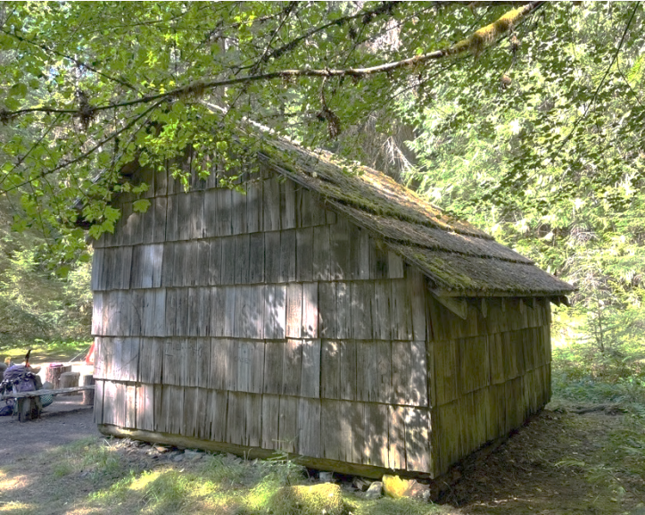
< North and east elevations showing vegetation encroachment
