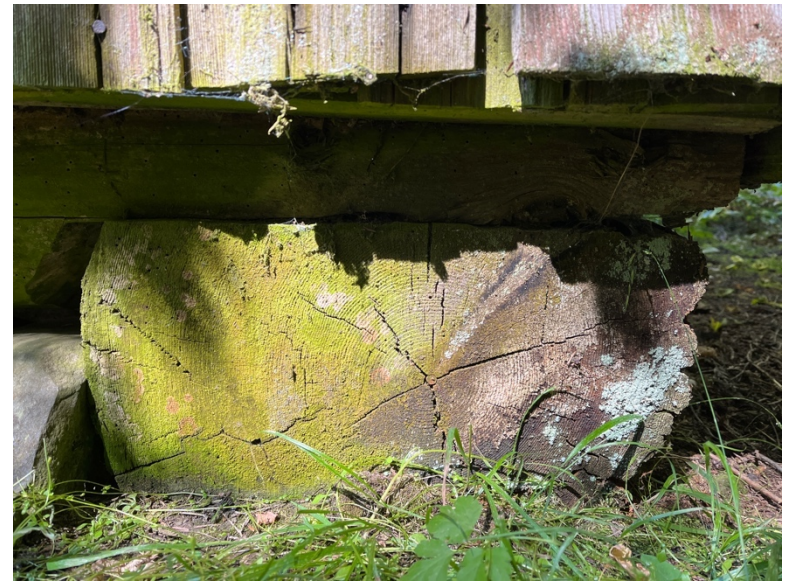
< End of sill log at ground contact; note extend of deterioration and what appears to be copper nail in the heart of the log
