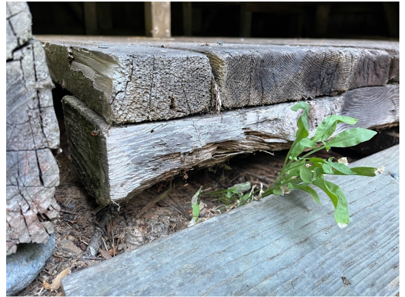
^ Detail of damage to SW corner floor joist
