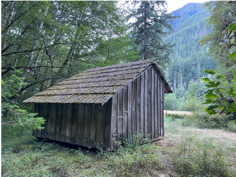
< North and west elevations. Note accumulation of debris on roof; note encroaching tree branches along east elevation
