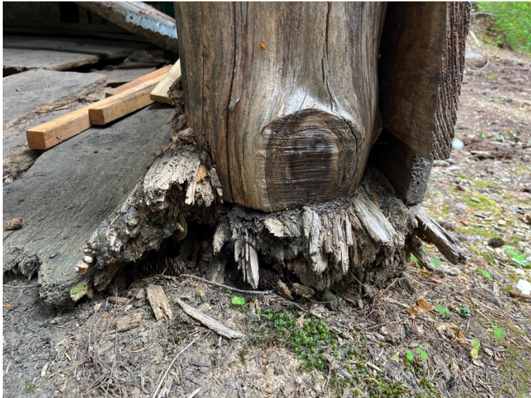
< Detail of sill rot on southeast corner
