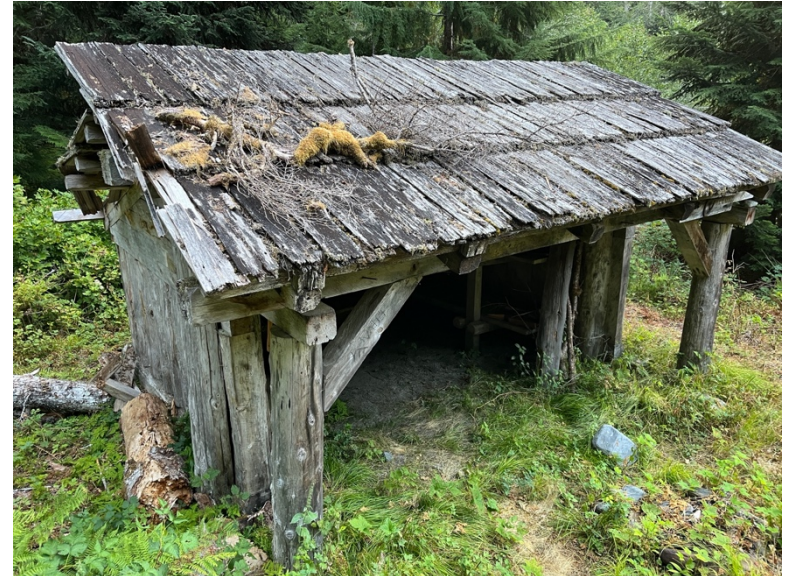
^ Detail of roof on south elevation; note encroaching vegetation and lack of adequate drainage around structure; accumulated debris on roof
