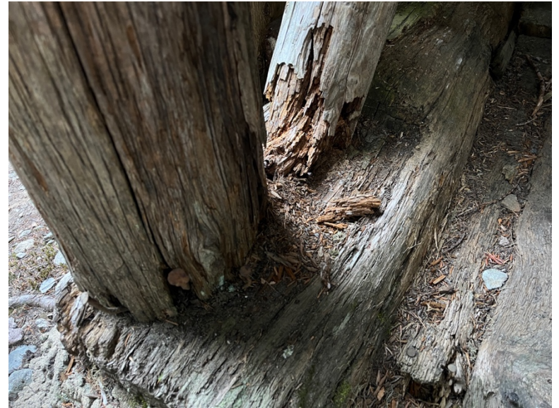
Detail of sill and post rot on southwest >
