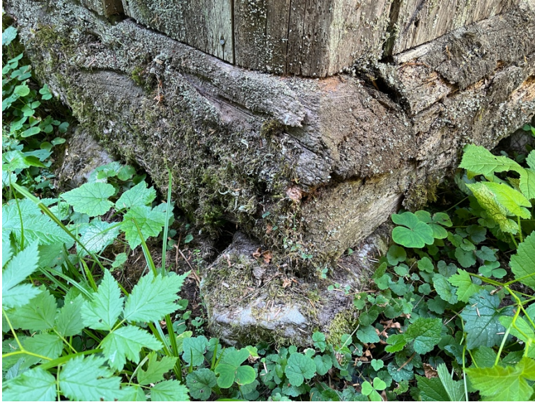
< NE corner sill log; example of deterioration found along extent of sill logs; note lap joint
