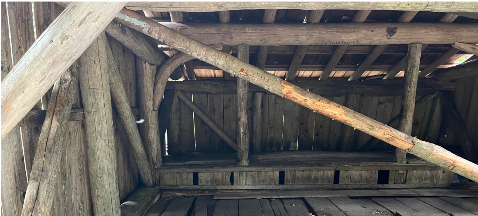
Interior of Anderson Pass shelter showing diagonal bracing log secured with metal strapping used to stabilize construction due to building's poor condition, 2022. Photo by author.
