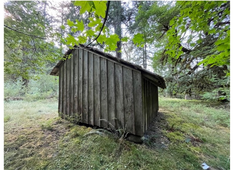
^ North and east elevations. Note encroaching tree branches.
