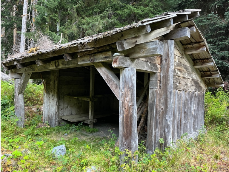
< South (primary) and east elevations showing vegetation encroachment on all sides including interior
