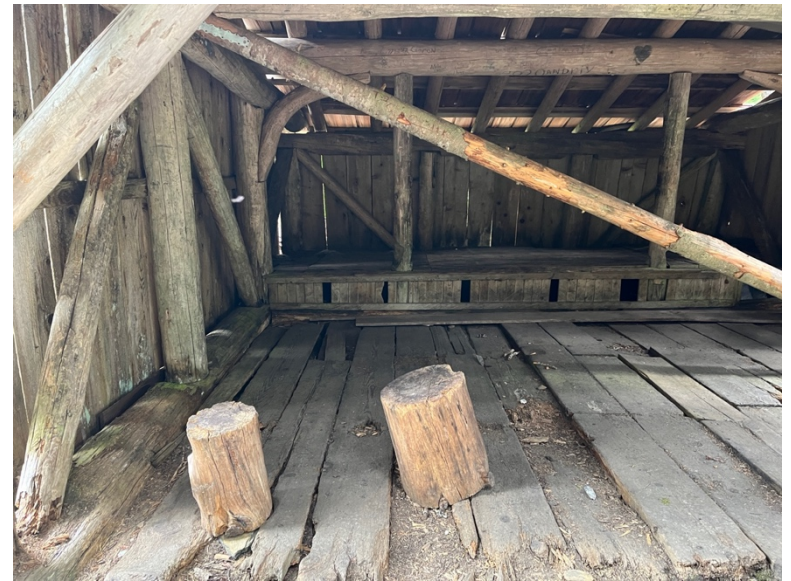
Missing or water damaged floor planks at southwest corner; note several missing siding from bunk structure >
