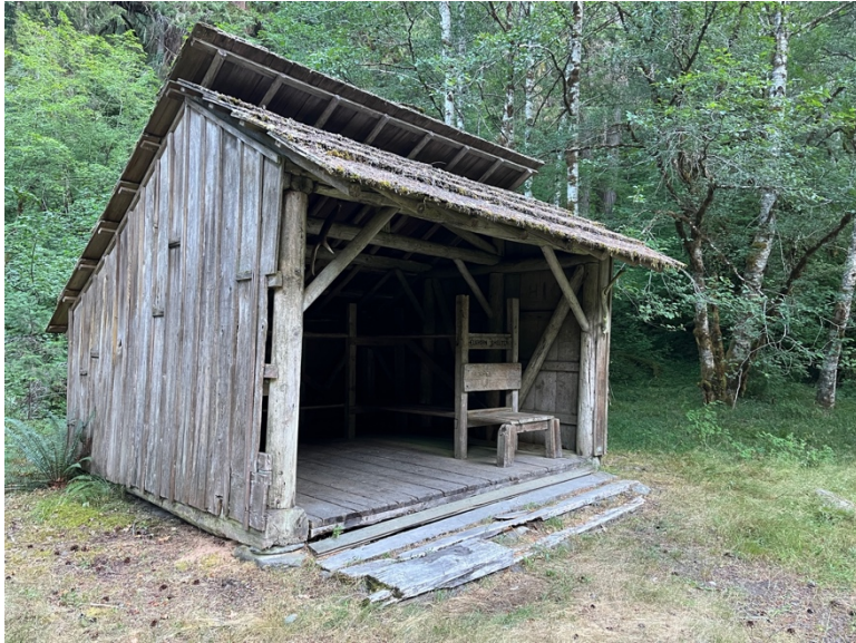
< West and South (primary) elevations. Note deterioration of exterior porch planks and half damaged siding board on SW corner
