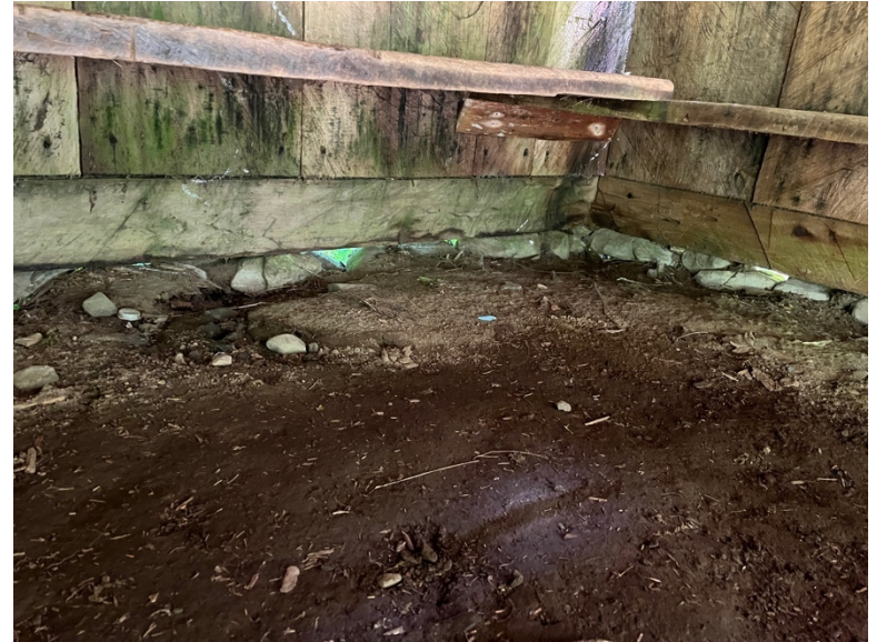
Evidence of moisture accumulation in interior >
