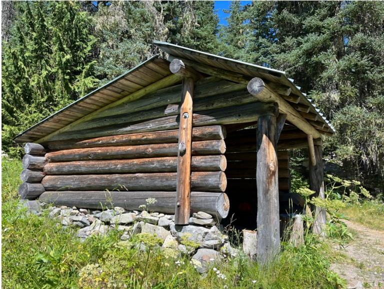
< West elevation showing extent of weathering on siding logs and condition of stacked rock foundation
