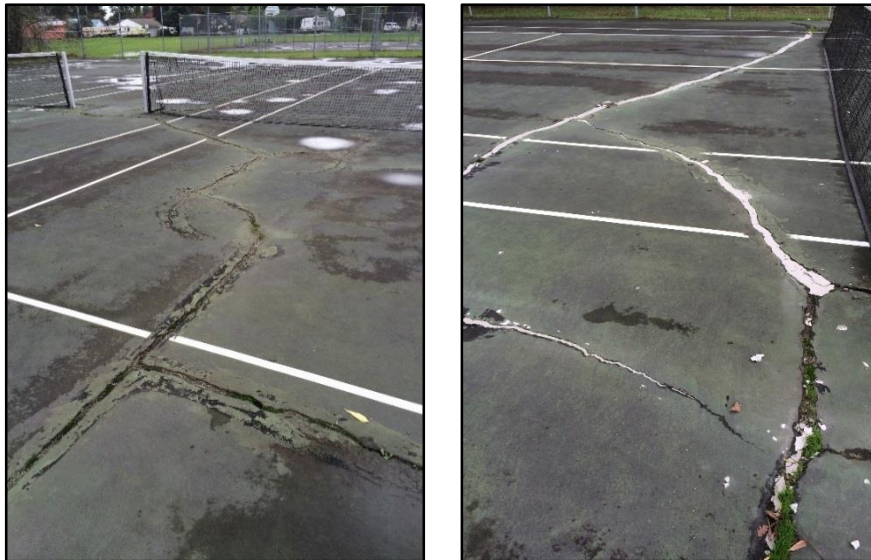
Tennis court cracks and previous attempts to repair cracks
