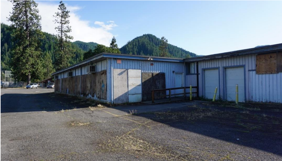
Figure 2: Current Condition of the outer east side of the WAC, 2025
