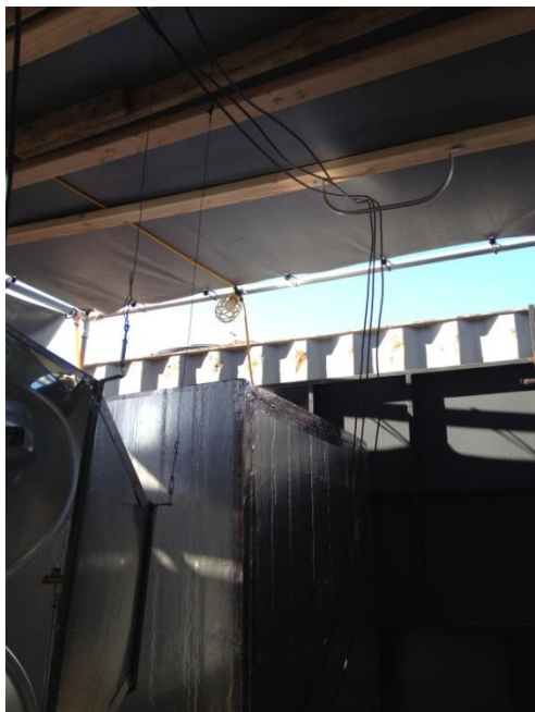
P30. Sensors travel from the data acquisition center (P1, P2) to various locations. Sensor lengths are 40-feet and provide ample coverage of the entire Solar Simulator and to Weather Station
