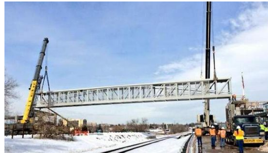
Tandem crane emplacing pedestrian bridge in Fort Collins, CO over BNSF Railway tracks. (Shelby, 2014)
