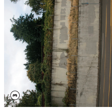
Remaining Wall Cutting off Circulation
