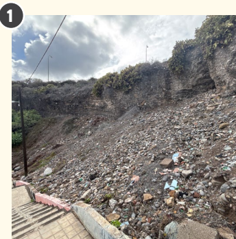
Steep, unvegetated slopes shed stormwater toward infrastructure downslope.
