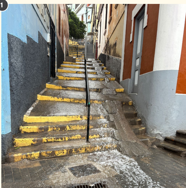
△ Calle Nogal Entrance: Stormwater accumulates in the public right-of-way at the bottom of the slope.
