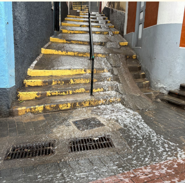
Calle Nogal, El Risco de San Nicolas: Runoff accumulation in the public right of way.
