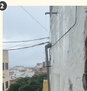
Rooftops drain directly onto pedestrian corridors.
