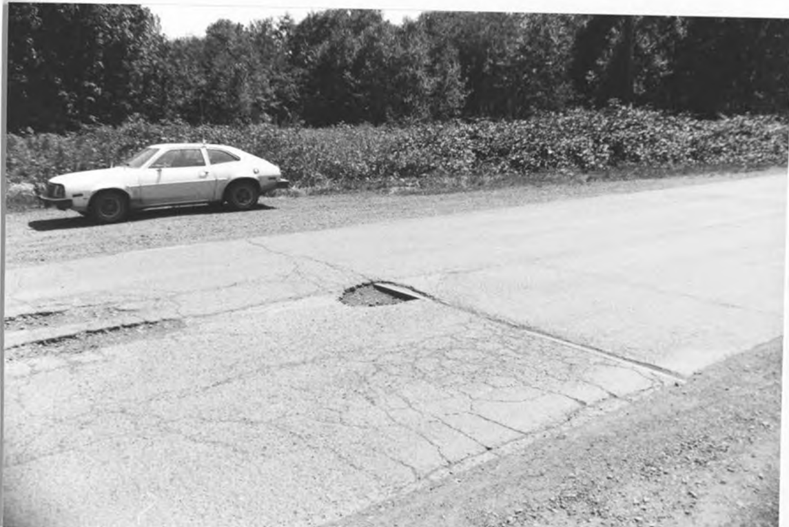
Figure 30: The rails of the old Salem, Falls City, and Western Railroad are visible through the cracking pavement of this Falls City street.
