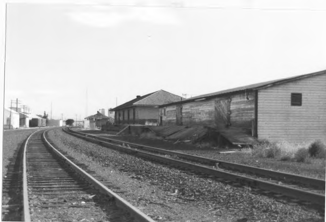
Figure 24: Although many industries still ship from the Redmond rail corridor, the presence in this neighborhood of abandoned structures such as this warehouse, with its collapsed loading dock, give the corridor a deserted, ghost-town appearance.
