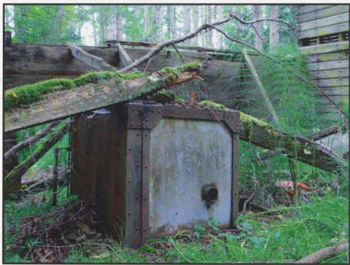
Fig.3.4 Nature has reclaimed the drier, especially failed interior components which have heavy moss accumulation. Photograph by author.
