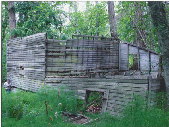
Fig.3.2 The Clark Prune Drier as photographed in 2010. Approximately 50 per cent of the drier is estimated to be lost or dislocated, including interior components and the roof. Photography by author.
