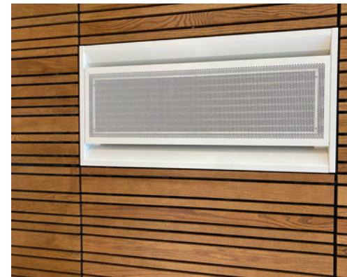
FIGURE 117 | HVAC/MEP of Tykeson Hall. (Aaryn Gray, 2022)
