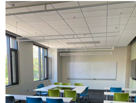
FIGURE 116 | HVAC/MEP of Tykeson Hall. (Aaryn Gray, 2022)
