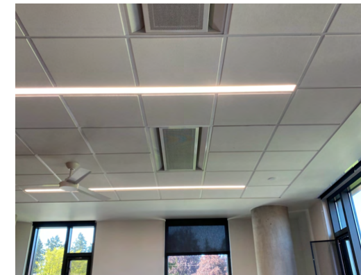
FIGURE 118 | HVAC/MEP of Tykeson Hall. (Aaryn Gray, 2022)
