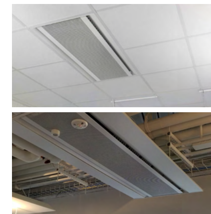
FIGURE 122, 123 | Pacific Chilled Beam, Installed. (Swaegon, Date Unknown)
