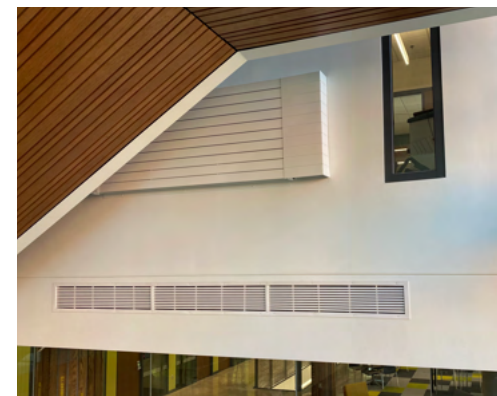
FIGURE 119 | HVAC/MEP of Tykeson Hall. (Aaryn Gray, 2022)
