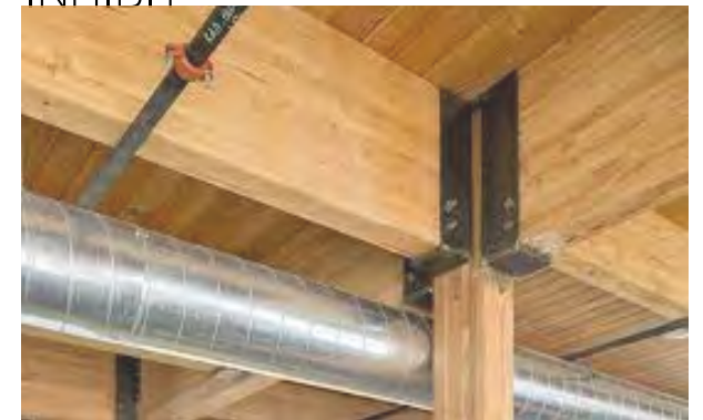
FIGURE 4 | Glulam Post and Beam with Ducting. Radiator Building, Portland, OR. (Josh Partee, 2017.)
