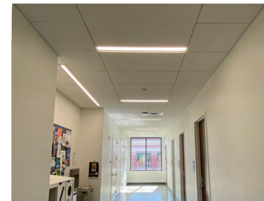
FIGURE 120 | HVAC/MEP of Tykeson Hall. (Aaryn Gray, 2022)
