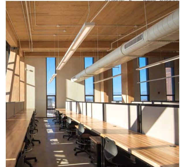
FIGURE 63 | Exposed Systems in Studio Classrooms. (Leers Weinzapfel Associates, 2015)
