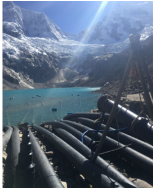
Figure 5: Glacial Lake Palcacocha with siphons installed to lower lake level. Photo by H. Moulton
