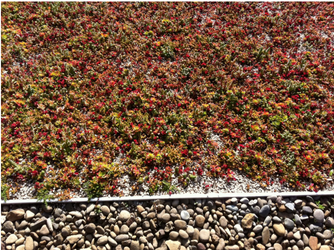
Ecorooftop for storm water management
