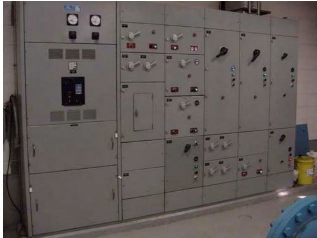
Motor Control Center
