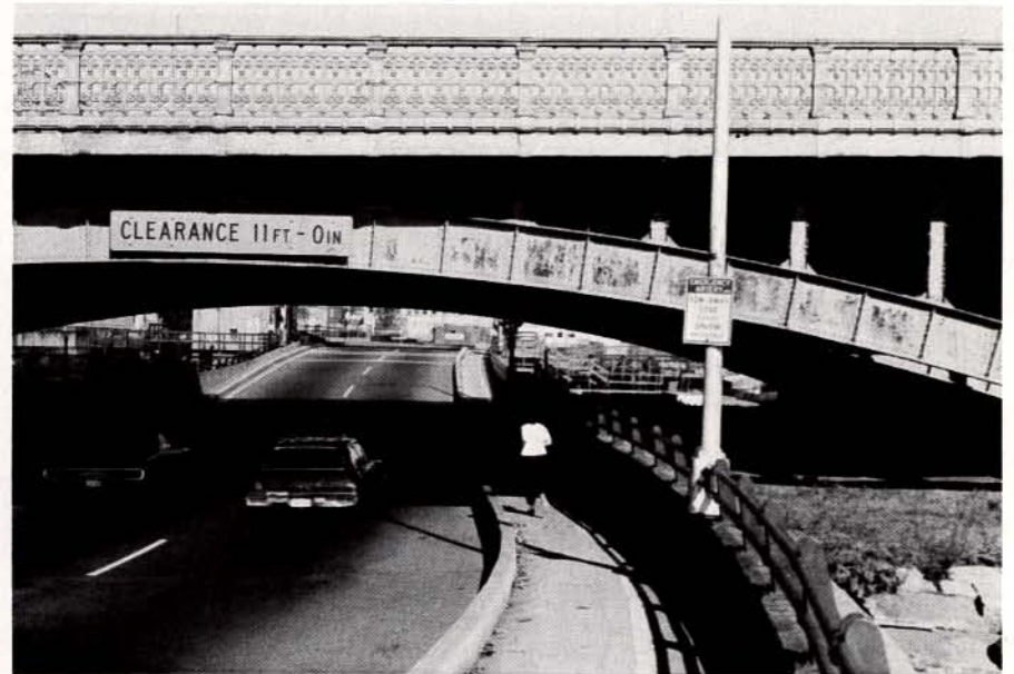
c. Traffic lanes were realigned for widened bike path under the viaduct.
