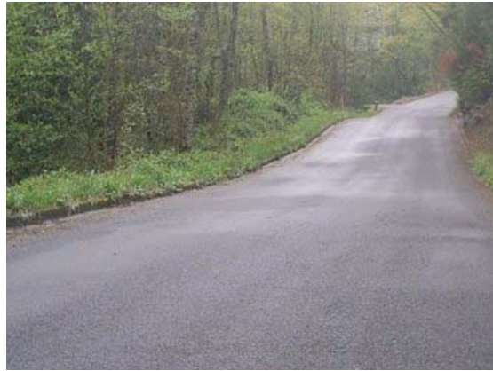
Soil creep: undulating pavement and curbs
