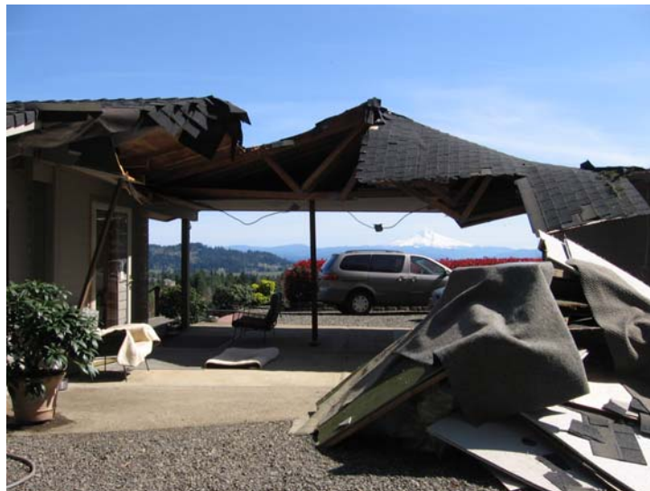
Damage to Damascus home from windthrown timber. This occurred during the December 2006 windstorms.
