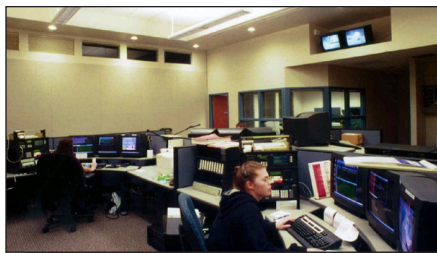
KITTCOM Control Center, Ellensburg. The only number you need to report a fire is 911 which will connect you directly to this control center.
