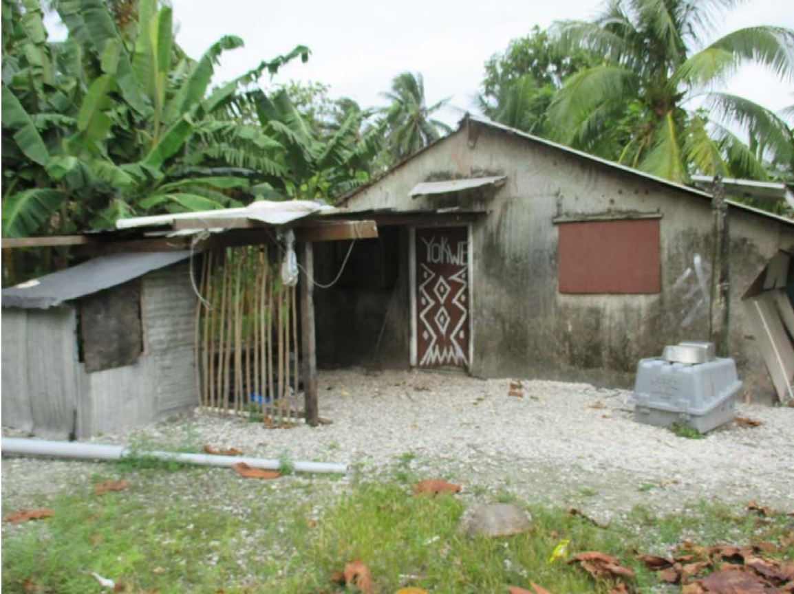
Figure 136. Photograph of a Typhoon Mon on Monak wēto , Namdrik. Note the cookhouse is attached to the front entry gable. Also, note the battered walls.
