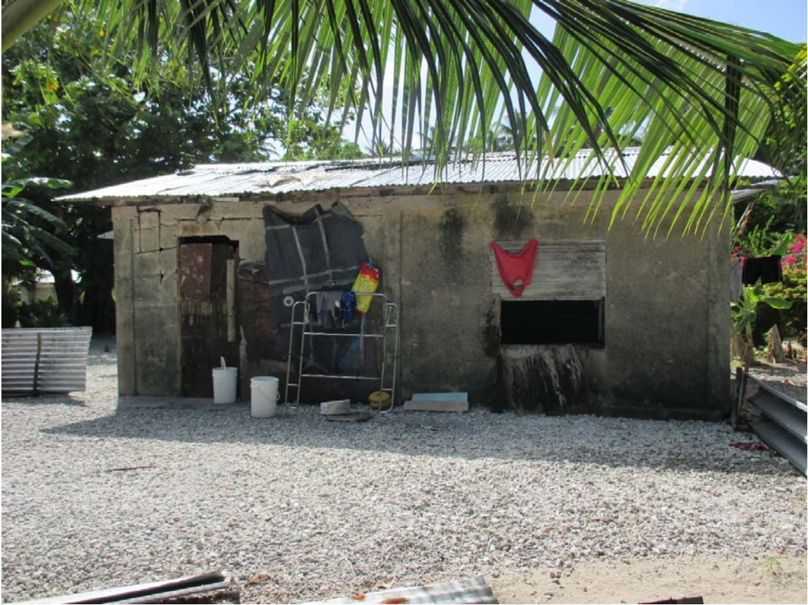
Figure 203. Photograph of house 'A' showing the damage created overtime from the harsh winds whipping the lagoon side elevation.
