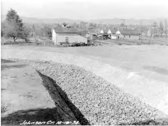
Work Projects Administration (WPA) Johnson Creek channel project in the early 1930s. City of Portland photo.
