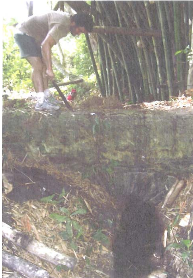
Figure 59. Bridge used in the acequias to cross-creeks or other acequias. Where the person is standing is the canal for the water, and on the arch at the bottom another acequia circulate. Hacienda Playa Grande. Photo by author, September 2009
