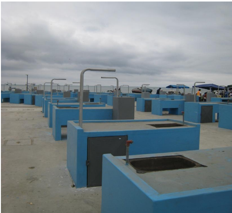
Image 12: New fish cleaning and vending stations built by Manta's government in attempt to help clean up Tarqui's beach. Though hard to notice in this picture, the sinks are already seriously rusted before they have even been used due to cheap building materials. (Author's photo)
