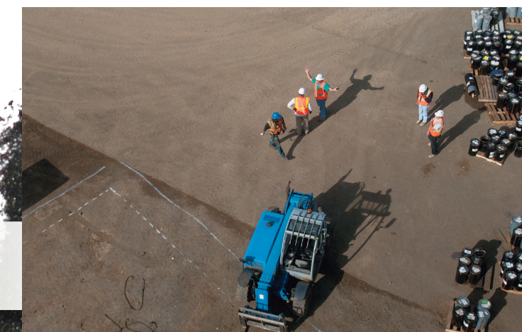
Workers building a chromite processing plant along the harbor, visible from downtown Coos Bay.
