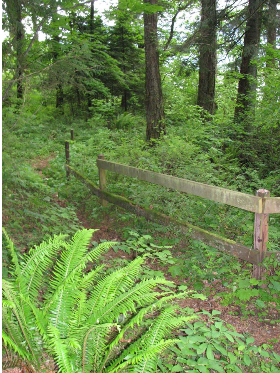
Figure 26. Buck Point Trail fencing, in poor condition. The trail runs along the northern portion of the campground, behind the campsites at the edge of a sharp dropoff. Recommended to either remove the fence completely where not absolutely required for safety, or replace with the decorative posts (campsite markers), and heavy horizontal boards, similar to the pattern seen for the Historic Columbia River Highway guardrails.
