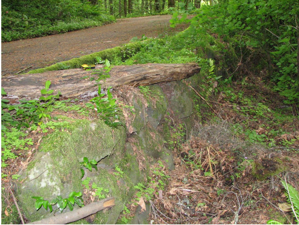
Figure 14. Civilian Conservation Corps-era rustic masonry retaining wall, near the entrance of the campground area.
