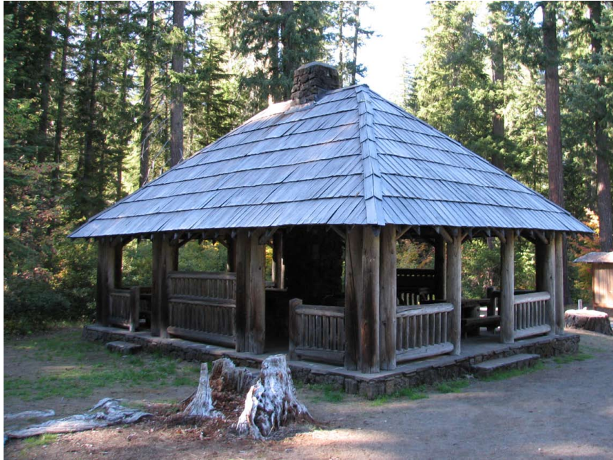
Figure 121. Civilian Conservation Corps community kitchen shelter, constructed 1935. Design from 1930s Recreation Plans Handbook, Plate 12-F) The structure is in good, overall condition, although the stoves need repair.
