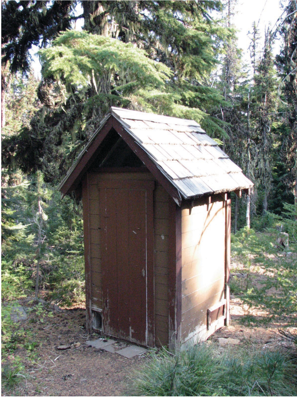
Figure 185. Guard Station toilet, likely constructed from Plate II or Plate II-A of the 1930s Recreation Plans Handbook.
