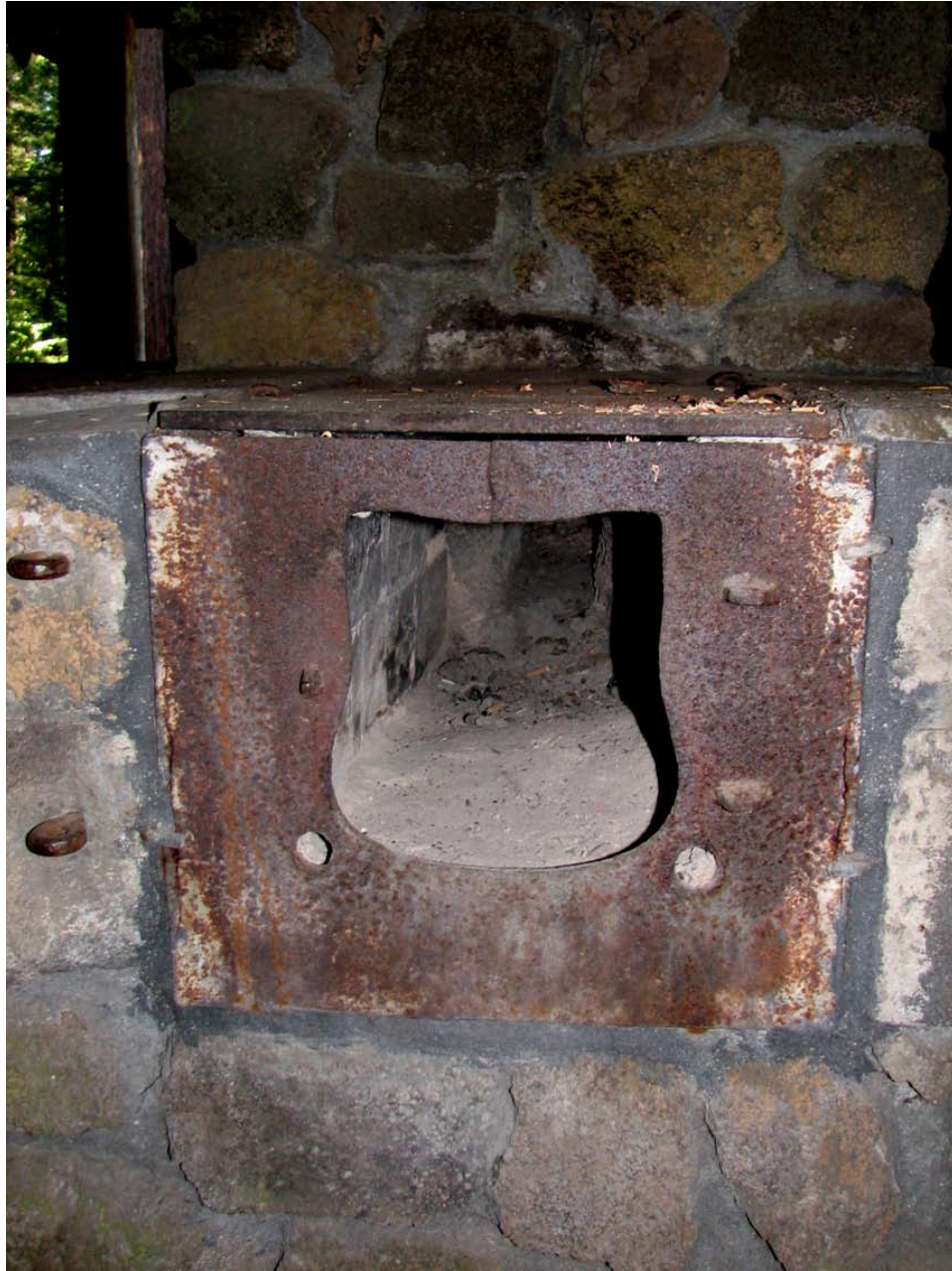
Figure 124. Community kitchen shelter stove example, needing firebox faceplate repair and replace missing door.
