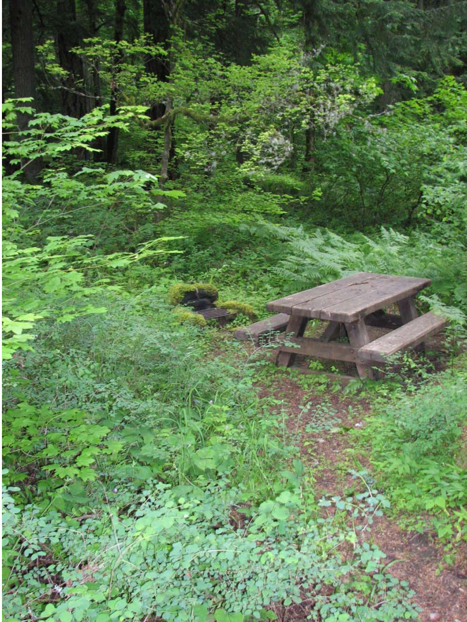
Figure 52. Lower area, picnic area and rustic fireplace. Fireplace in fair condition and requires repair.
