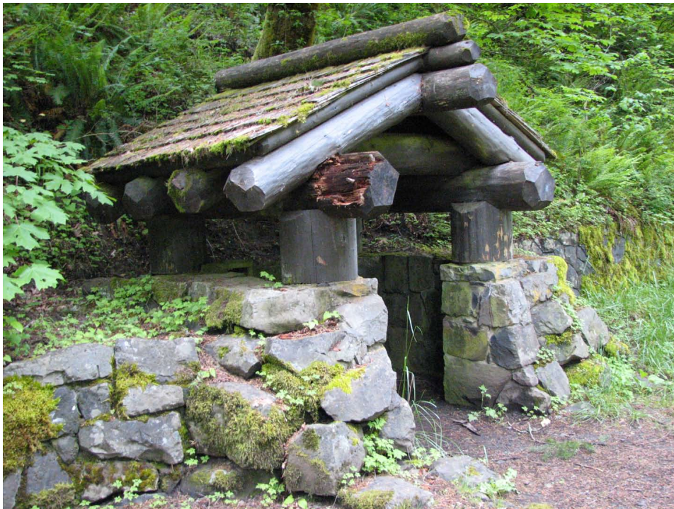
Figure 47. Lower area, Civilian Conservation Corps-era hiker register. Note fair-poor condition of support log. This must be repaired or replaced with in-kind materials.
