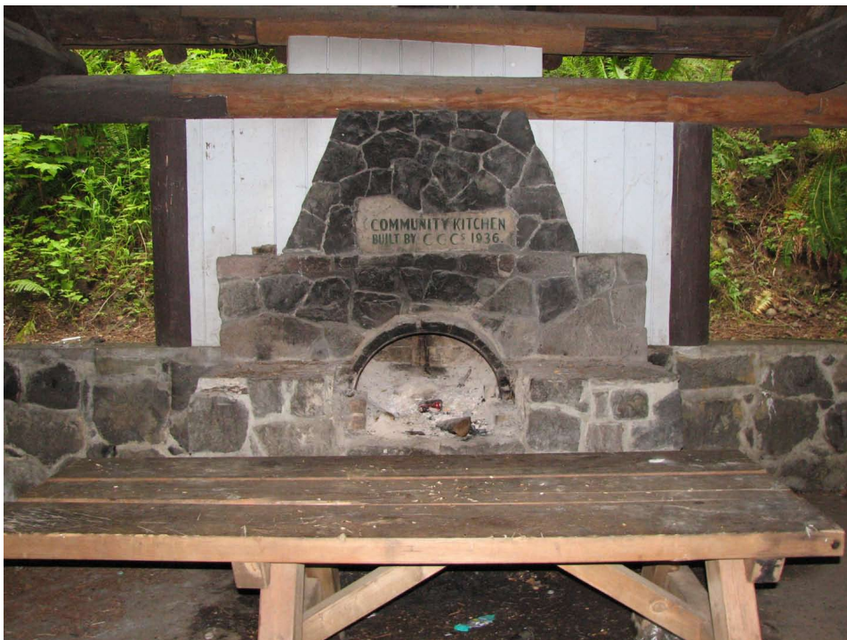
Figure 43. Lower area, showing community kitchen shelter recent repairs. Further research needed on white-painted wood surrounding chimney. This should be removed if not historic.
