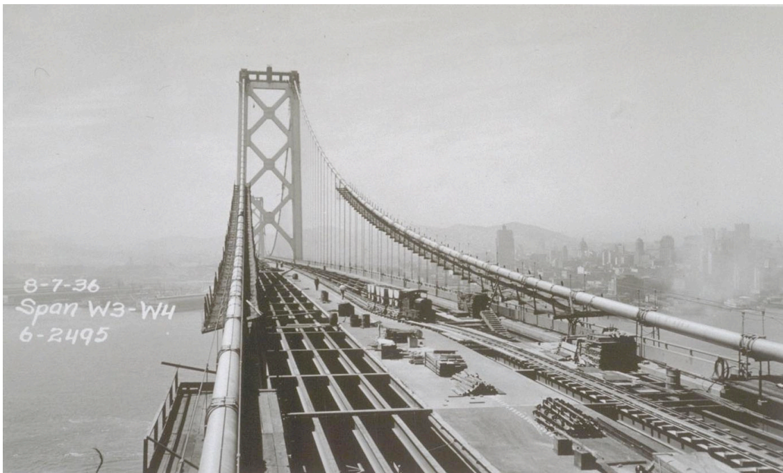
Figure 15: Construction of the San Francisco-Oakland Bay Bridge, 1936. Image courtesy of the Bancroft Library, University of California, Berkeley.
