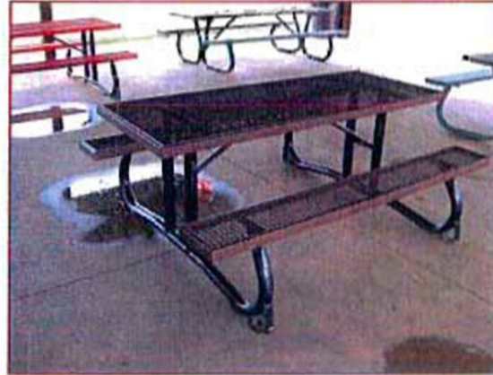
Figure 8. Large group shelter with visible puddles
