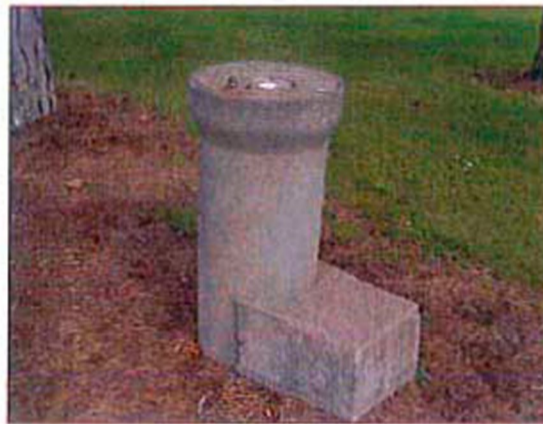
Figure 5. Damaged, non-ADA compliant drinking fountain
