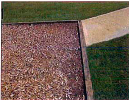
Figure 14. Playground access requires ramp for ADA compliance
