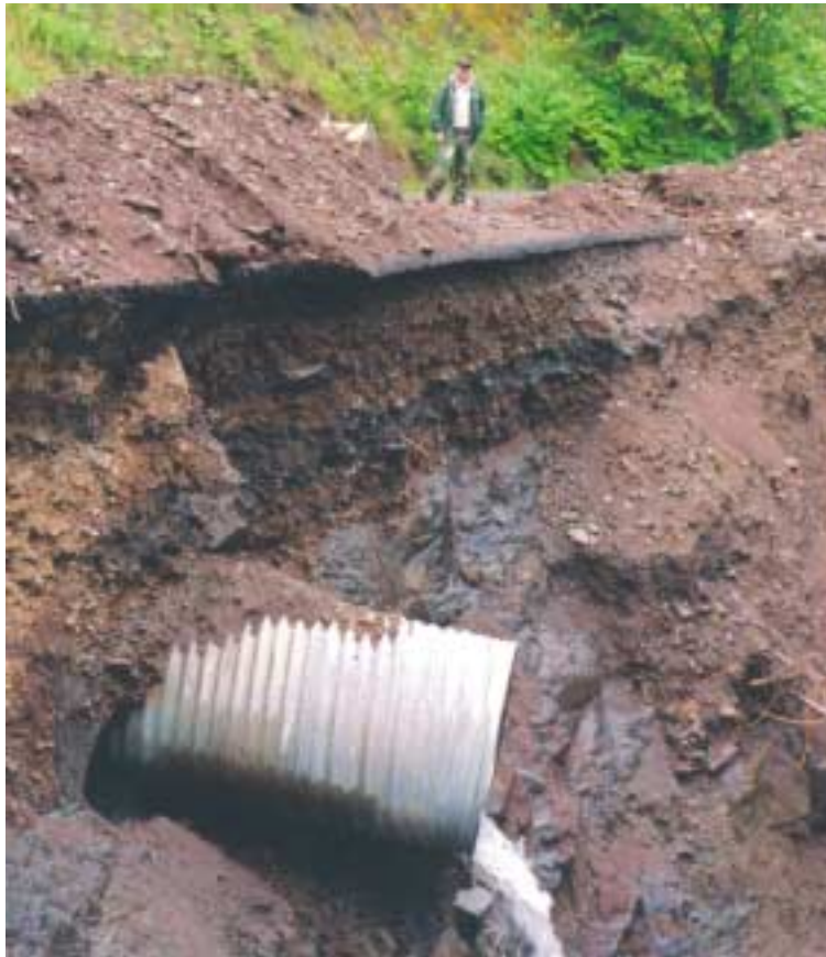
Figure 2. Effects of land movement on Forest Service Road #57. Note: This is the second time in two years that this road, just uphill from the mines has been forced to close due to major landslides. Photo by author.
