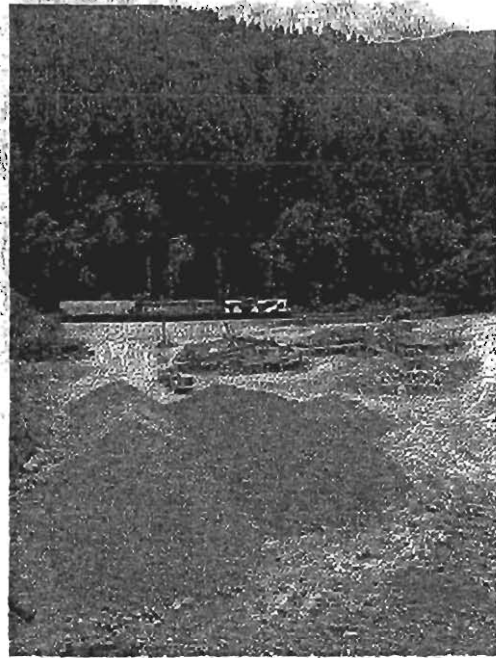
Overview of the distribution area with rock crushing equipment and piles of finished product ready for transport.
