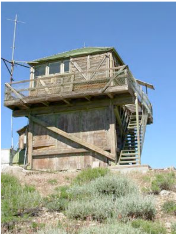
Figure 53: The Frazier Mt. Lookout was built in 1941 and has become dilapidated. In its current condition, it is very susceptible to an ignition from a wildfire. Windows are broken and holes are open in the wooden exterior. There was a piece of burned wood found on the ground that looked as if someone was trying to start a fire.
