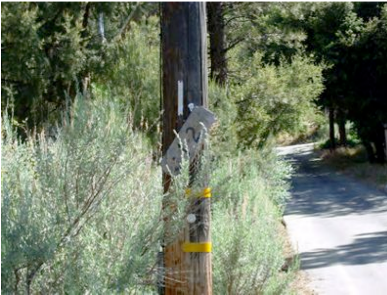
Figure 33: Example of an address sign posted in Pine Mt. Club that is ready to fall off the telephone pole. Besides the poor mounting, two of the numbers are missing from the sign that make finding the address difficult.
