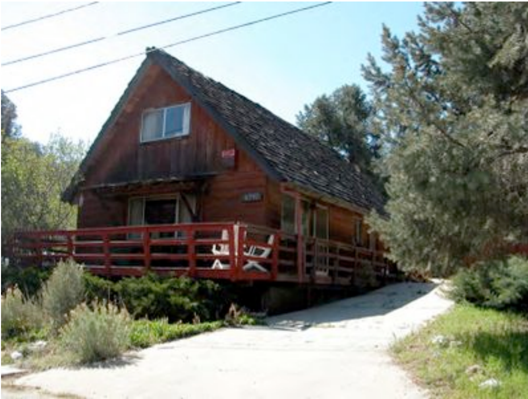
Figure 31: This home in Lake of the Woods would prove difficult to protect during a fast moving wildfire. The owners have chosen to use juniper to landscape and it is placed next to and under a wooden deck. The home is covered with wood shakes that burn readily and may spread fire throughout the area once they separate from the roof assembly.
