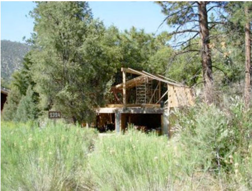
Figure 30: This home under construction in Pine Mt. Club is vulnerable to a wildfire. Notice the lack of clearance in the vegetation that makes defending this structure nearly impossible.
