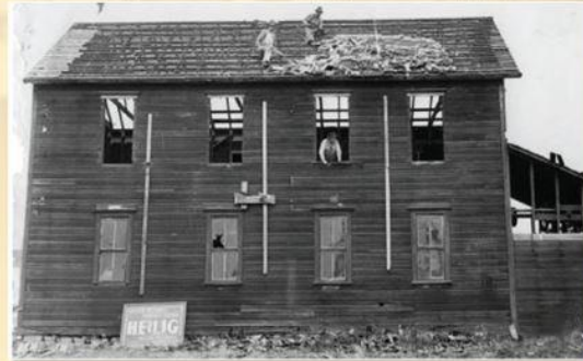
Razing the Barr Bros. Factory. Photo provided by Lane County Historical Museum
