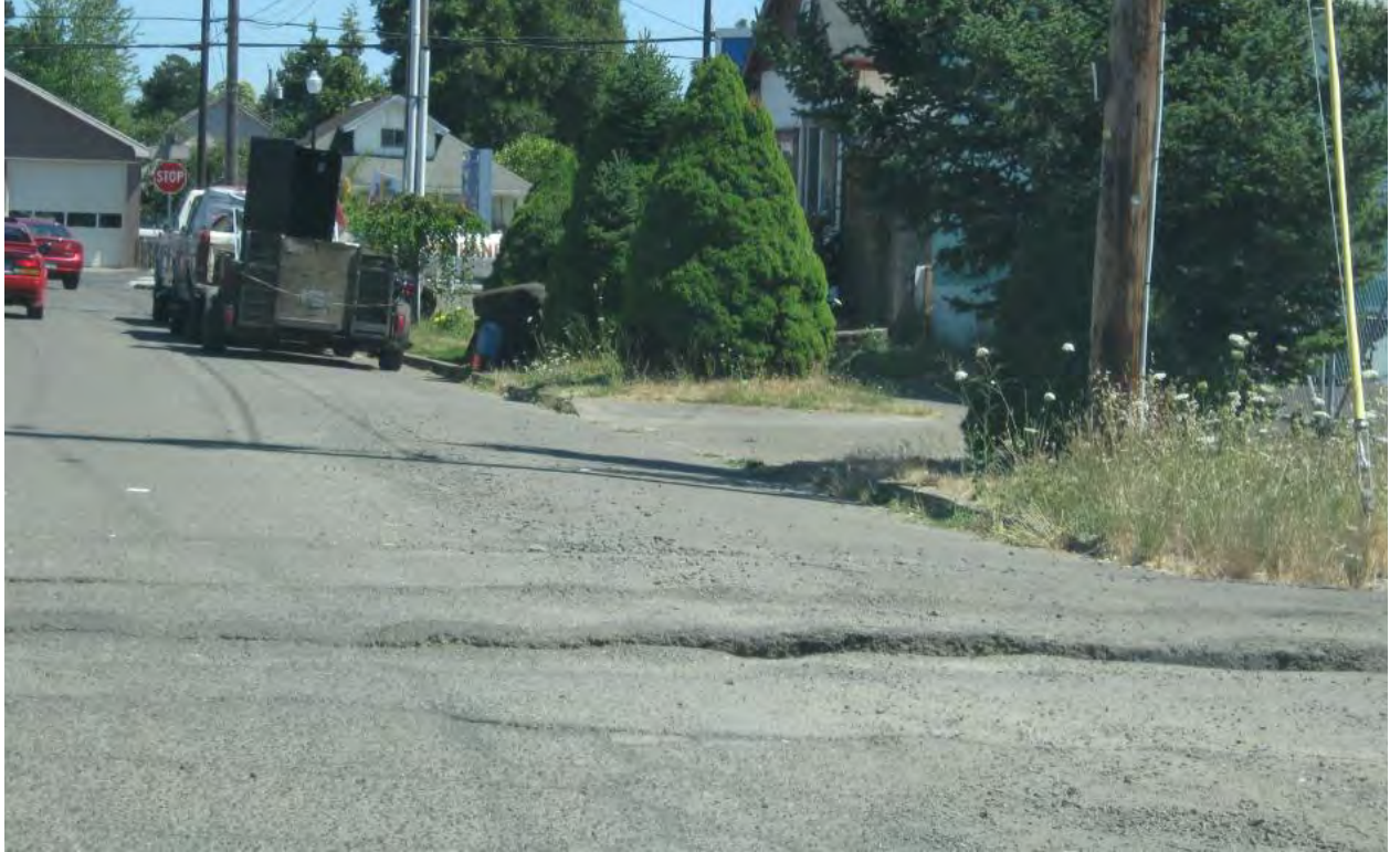
Deteriorated railroad crossing on 4 th Avenue, looking east.
