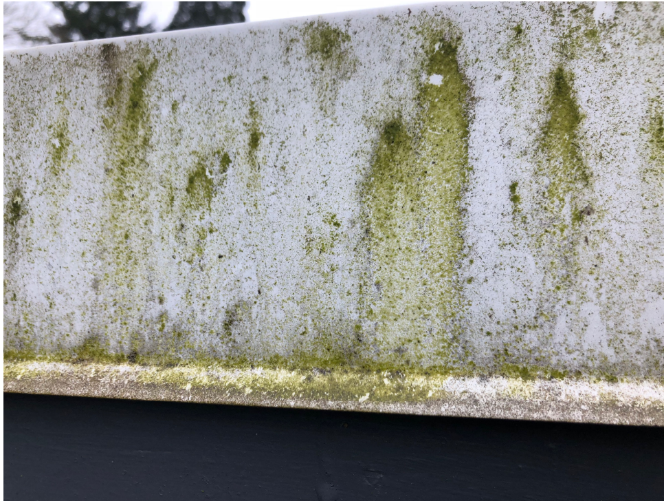
Figure 16 - Biogrowth along cornice, north façade.
