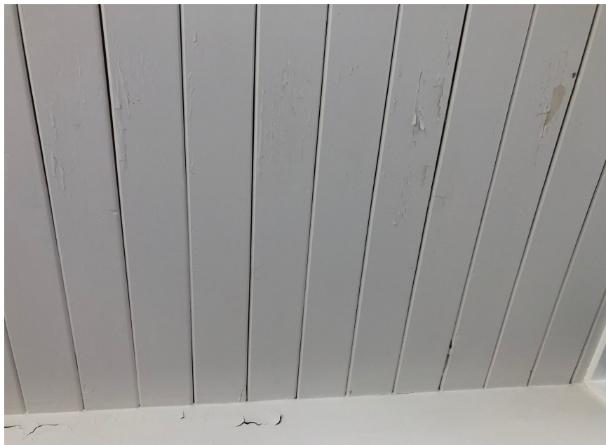
Figure 23 - Ceiling and top of wall, northeast corner of front bedroom.
