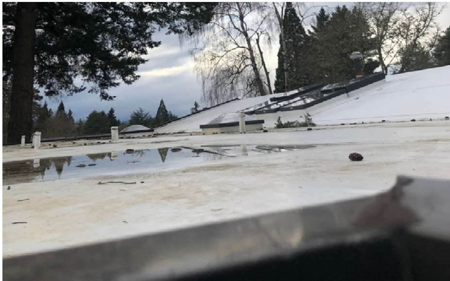
Figure 34 - Skylights and pooled water from poor drainage on roof, south façade facing north.
