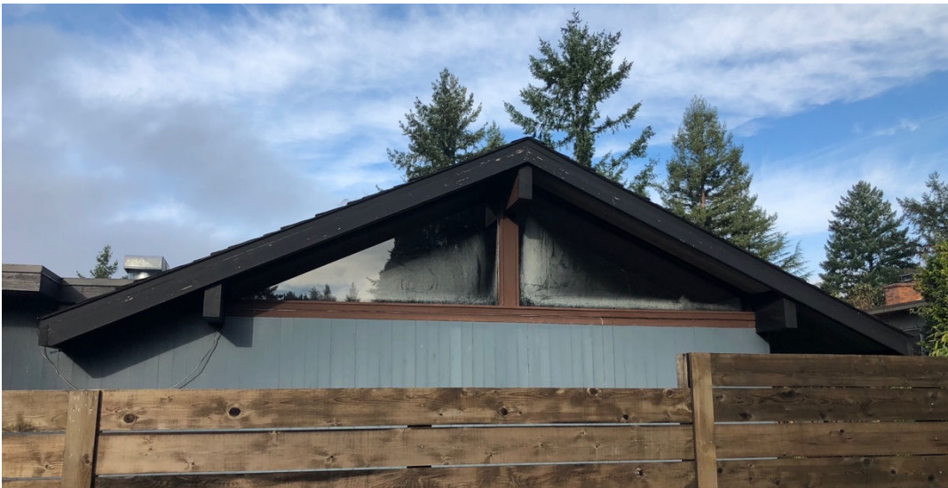
Figure 59: Condensation in a clerestory window of a Rummer house in an offshoot of 84th Avenue, facing north (Samantha Gordon, November 27, 2017).
