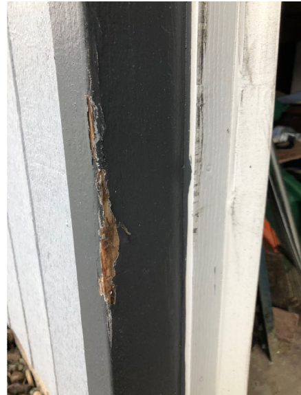
Figure 21 - North garage door frame damage detail, west façade.
