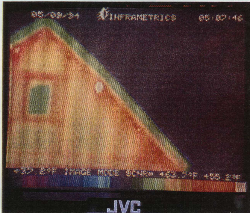
Figure 4-13 Exterior View of Heat Loss through Panel to Panel Joints, Fresh Air 80 Vents, and 2nd Floor Framing
