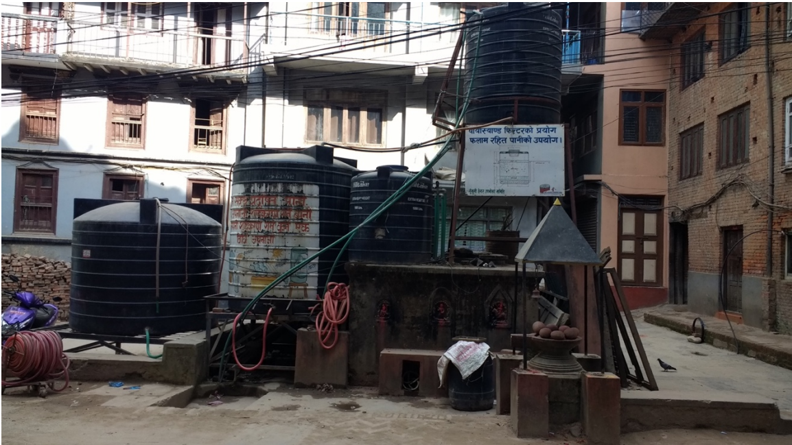
Figure 25. Local distribution tanks with a filtration system.
