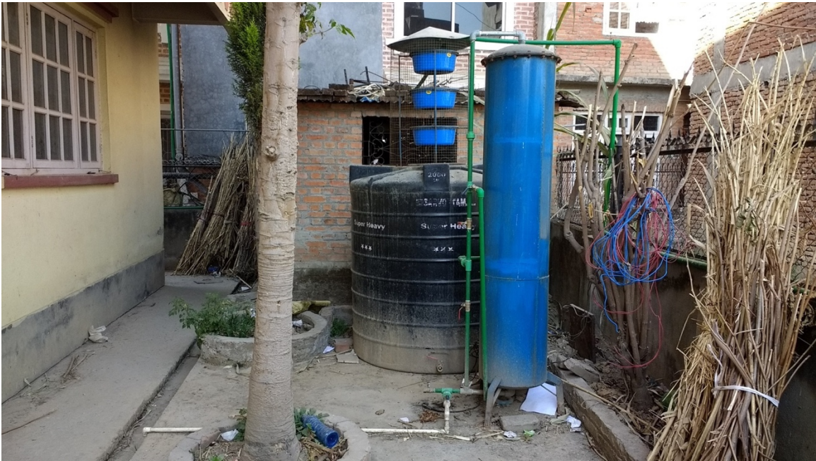
Figure 32. The household water cycle: Well water passes through the new filtration system before being pumped into her underground reserve and then to the rooftop tanks for use.
