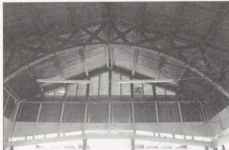
Fig. 22. Interior of clerestory showing the slightly sloping flat roof, plywood shutters in original openings, gable end louvers and roof sheathing. Photograph by author, 2008.
