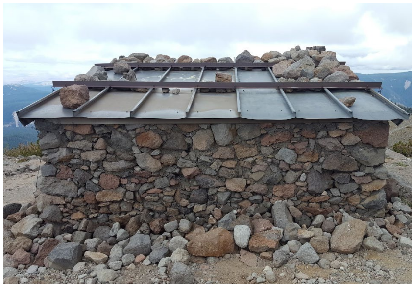
Rear wall condition and missing stones, 2017
