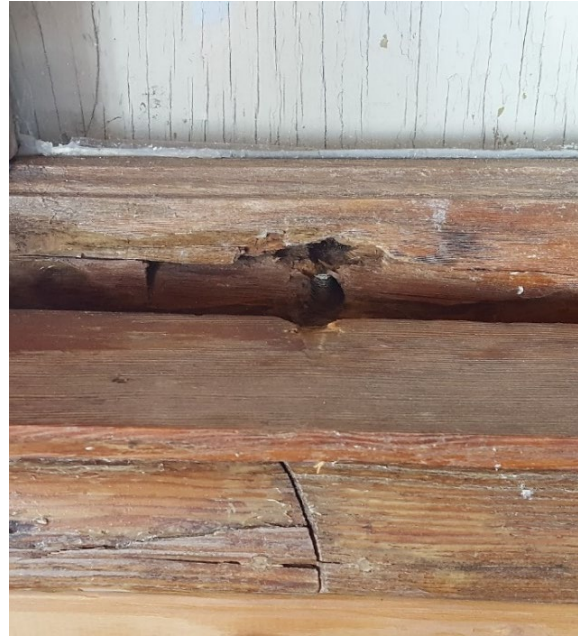
Condition caused by eyebolt installed through sash
