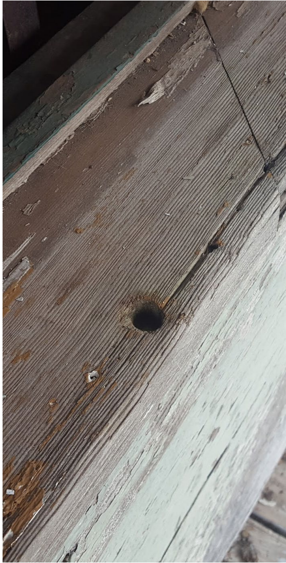
Typical condition, window sills
