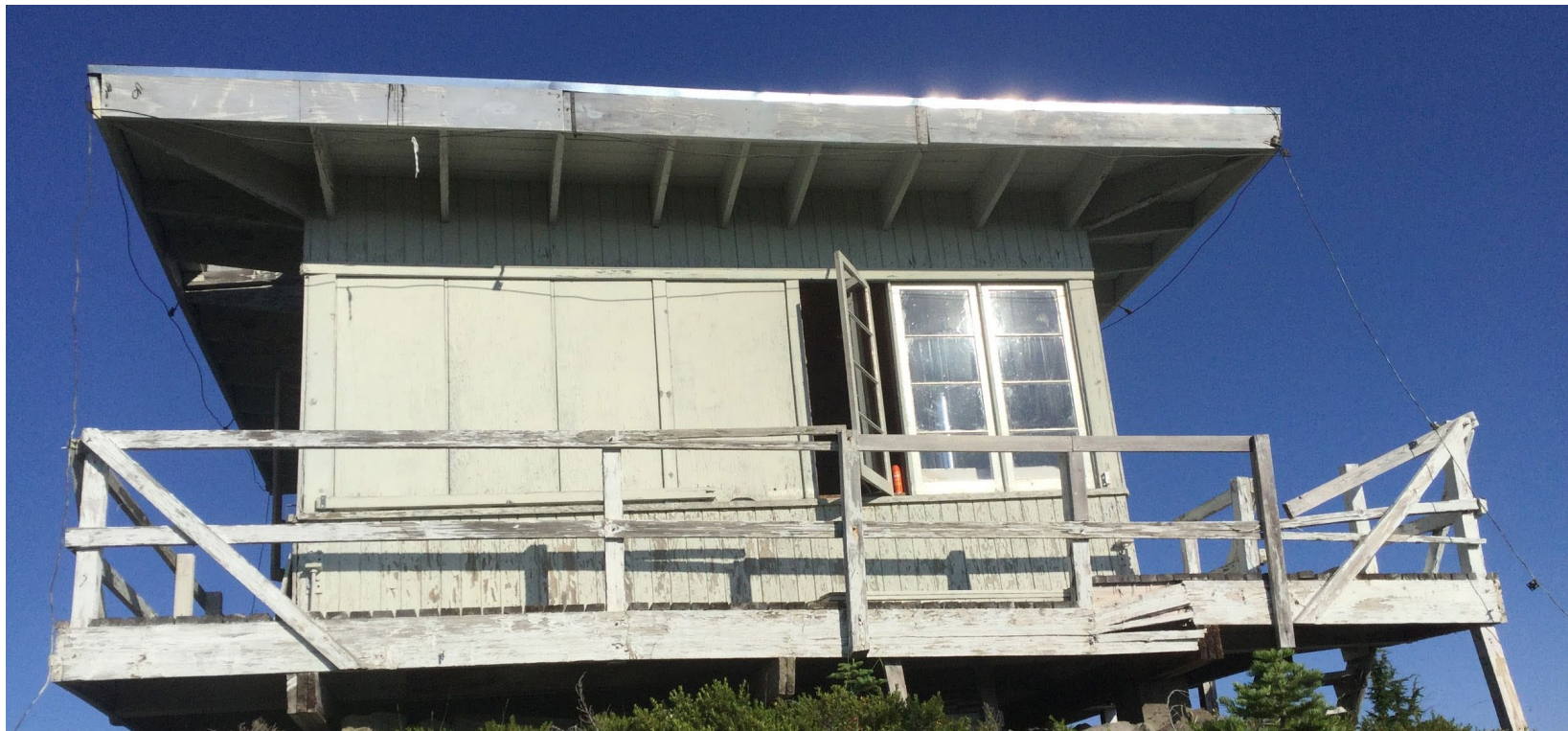
Unsecured window and broken catwalk on the east elevation present concerns about safety and security. Courtesy of John Milliken.
