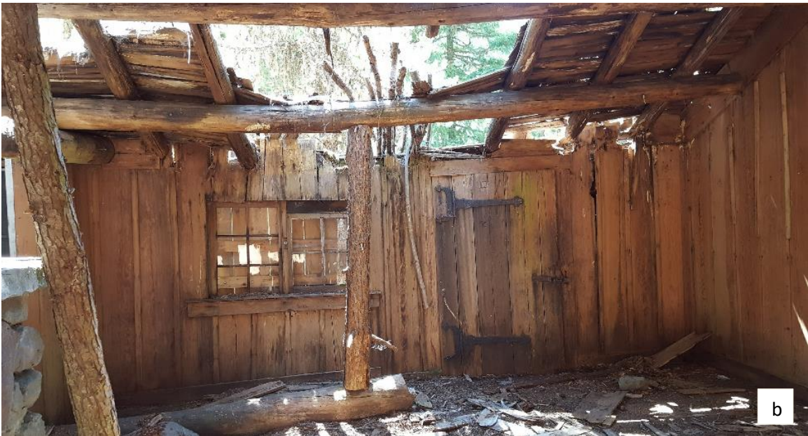
Figure 5.3. Exterior (a) and interior (b) views of the Upper Sandy Guard Station in the Mount Hood Wilderness, Mount Hood National Forest in July 2017. This building exemplifies the correlation between no active use (administrative or otherwise), no maintenance, and poor conditions.
