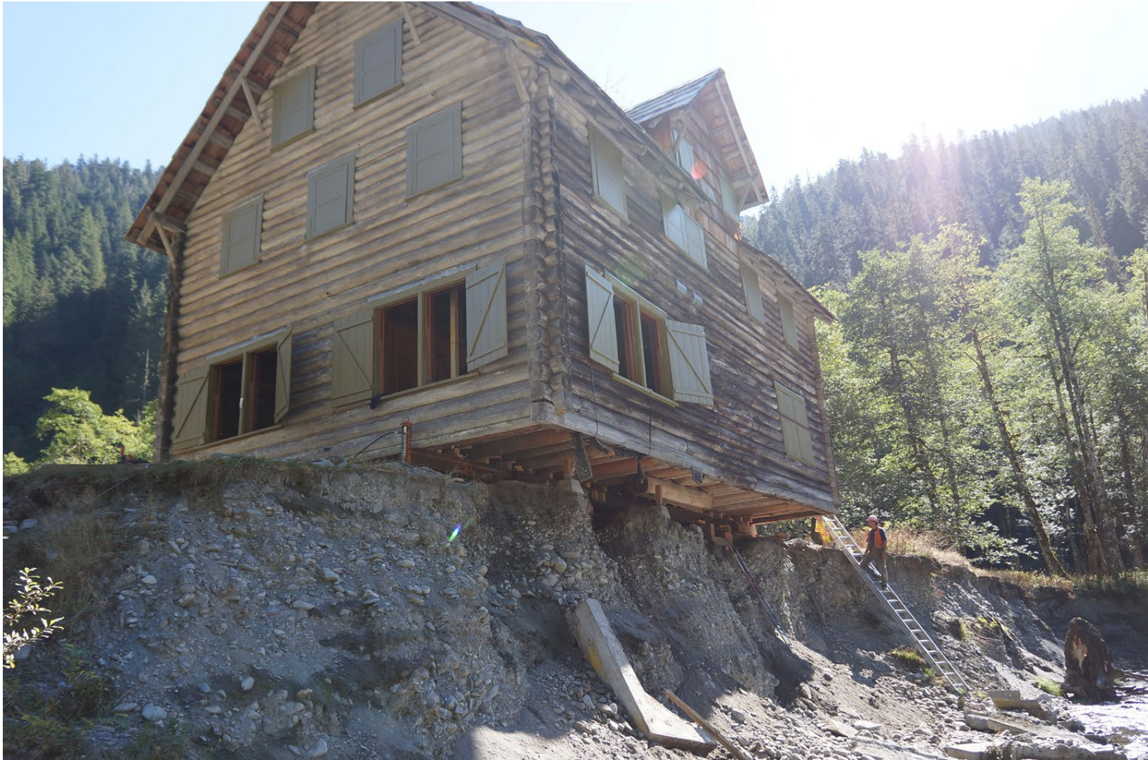
Figure i. The historic Enchanted Valley Chalet in the Olympic Wilderness of Olympic National Park, Washington, during a project to relocate the building away from an eroded bank of the Quinault River in 2014.
