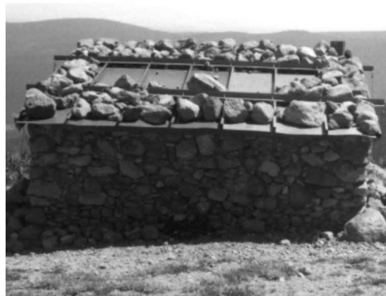
Rear wall condition, 1978. Courtesy of USFS
