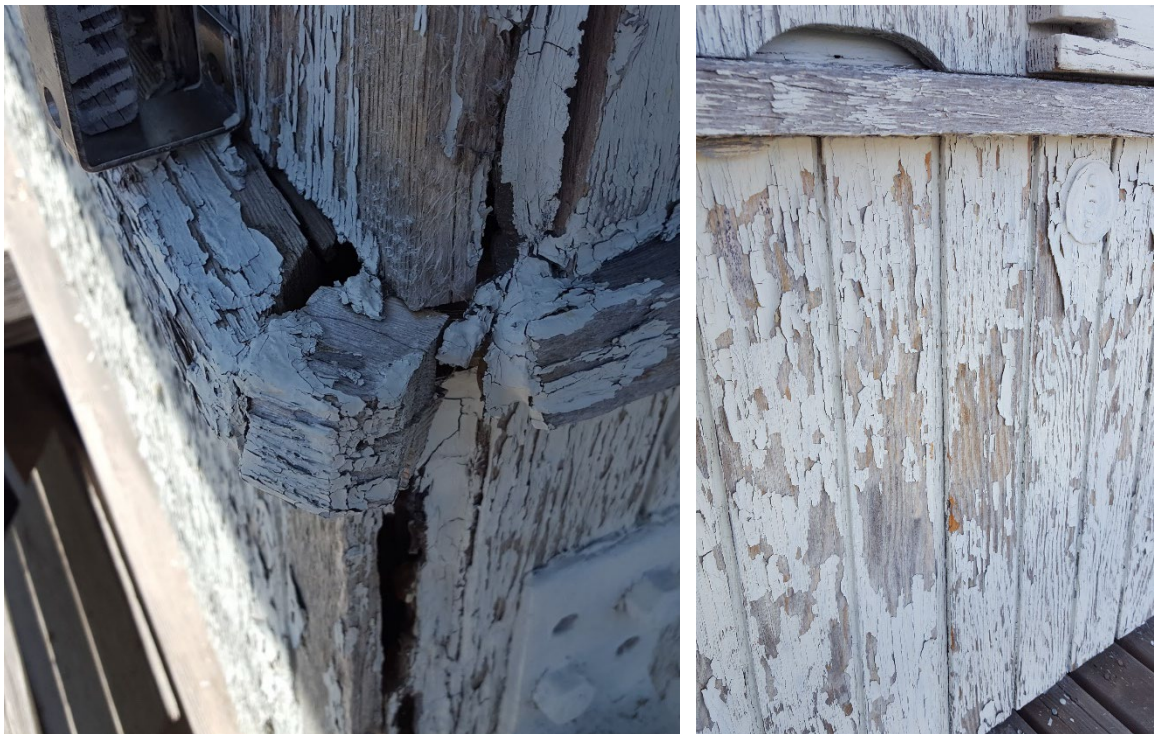
Figure 8. Photos of specific damage versus typical conditions
