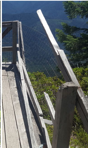
Broken northwest railing
