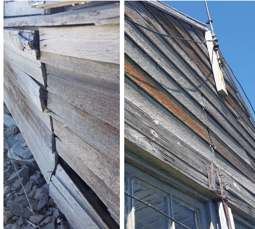
Typical condition below and above windows
