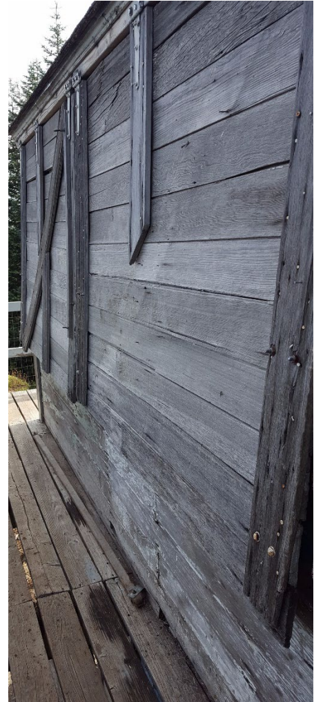
Condition of east shutters
