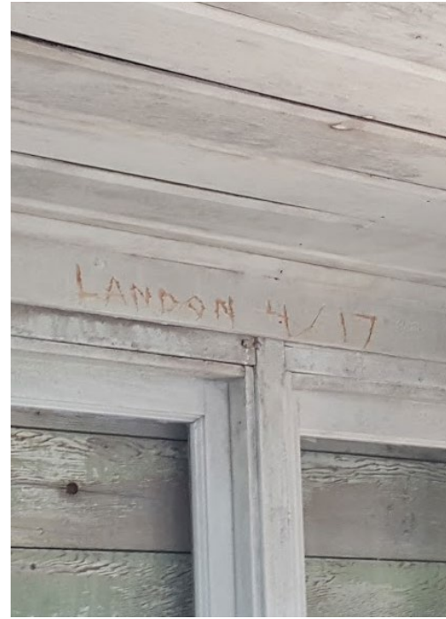
Carved graffiti damage
