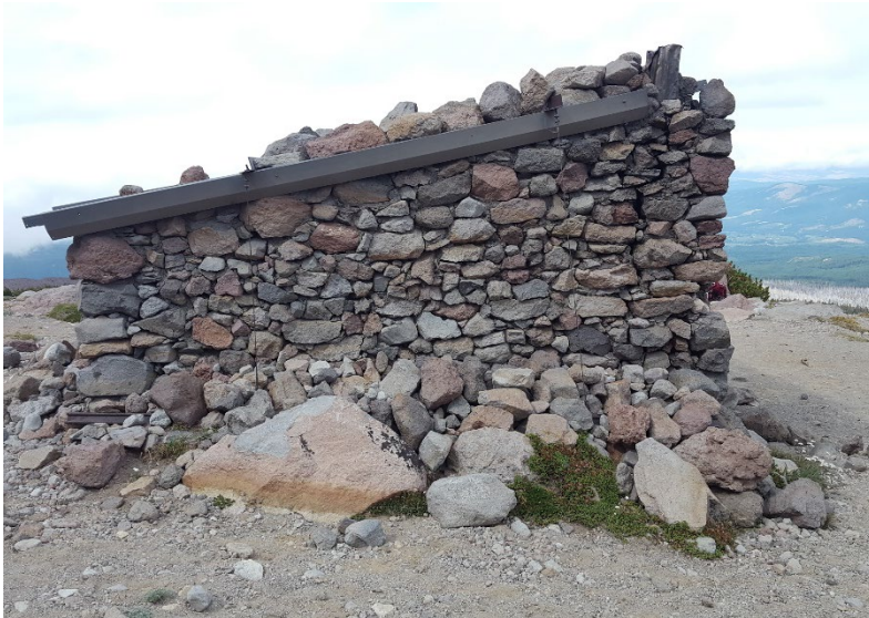
South wall condition and vertical crack, 2017
