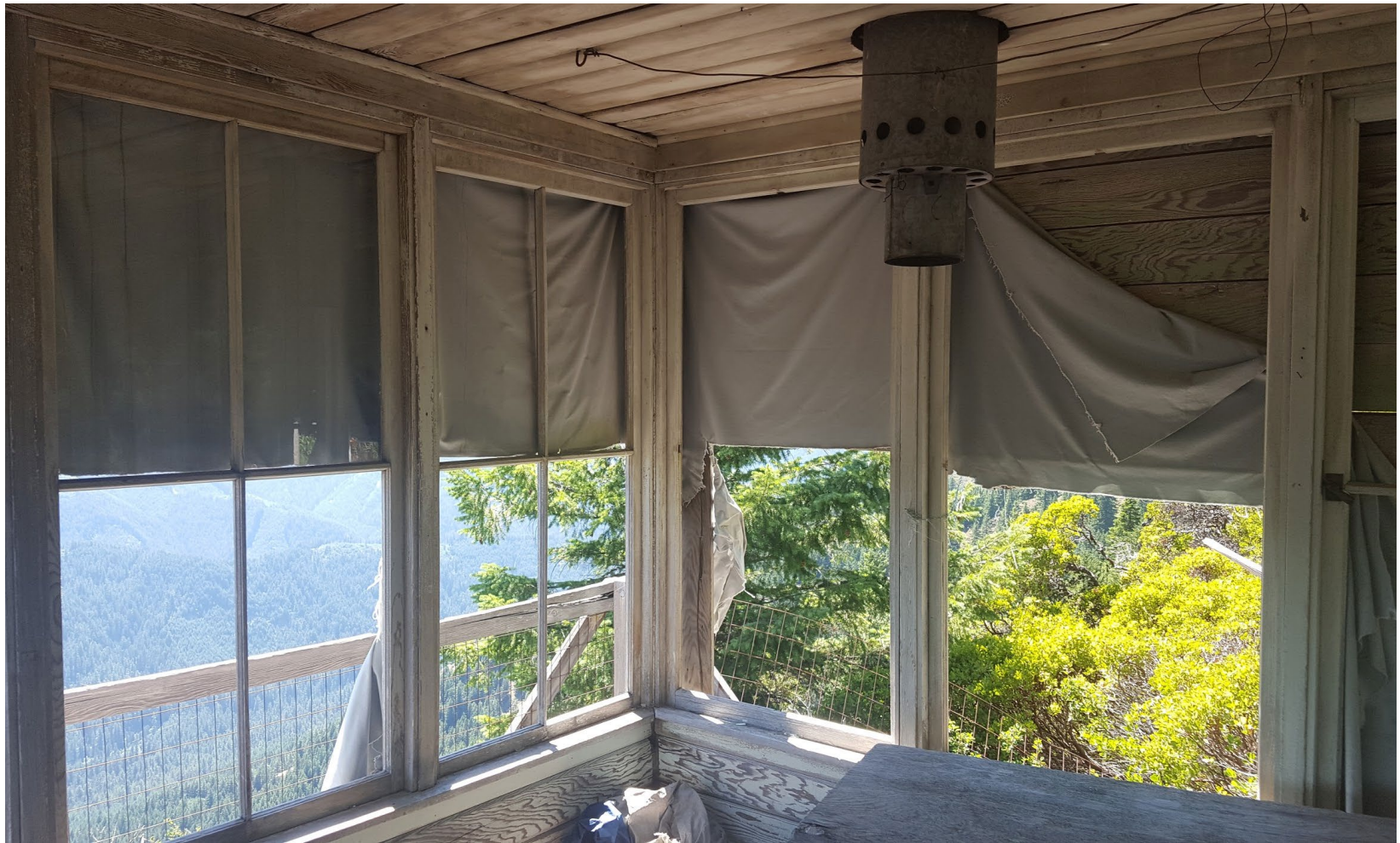
Windows in poor condition, with broken panes and muntins
