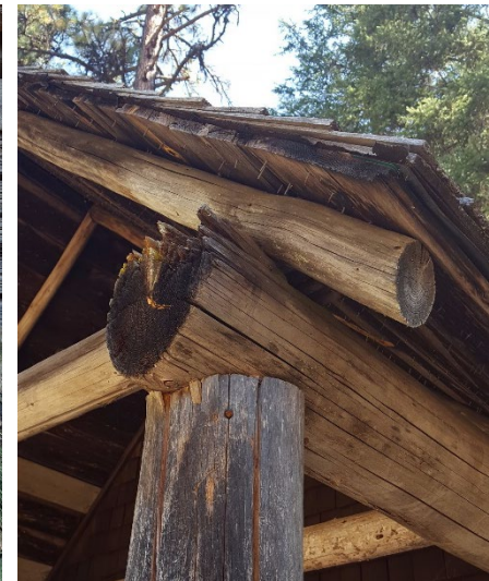
Condition at southwest corner
