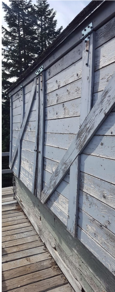
Condition of south shutters
