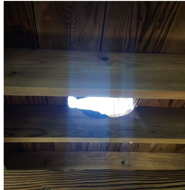
Burn damage, southwest corner
