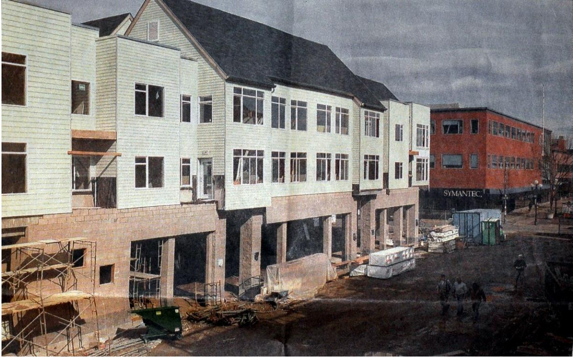
Figure 11.19. An image of Broadway Place Apartments under construction (sc. Register Guard March 21, 1999).
