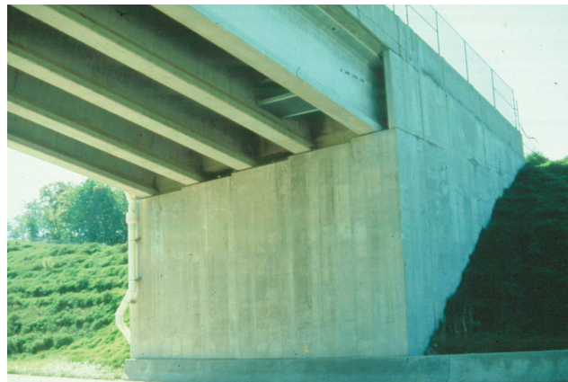
Figure 3.4: Example of concrete bridge abutment with wing walls. Source: 2012 FHWA Bridge Inspector's Manual
