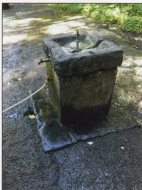
Figure 5. US 26 fountain with bad concrete patch.
