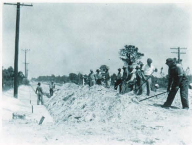
Figure 3: FERA workers constructing Bay Shore Road in Tampa, Florida. Photo Courtesy of State Library & Archives of Florida.
