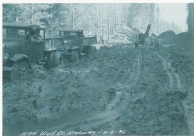
Figure 8: WPA workers constructing Wolf Creek Highway. Photo courtesy of City of Portland Archives.
