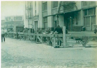
Figure 10: Sewer repair in downtown Portland. Photo courtesy of City of Portland Archives.
