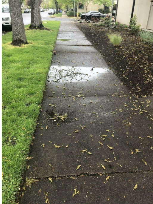
Figure 7. Flooded sidewalks on Patterson
