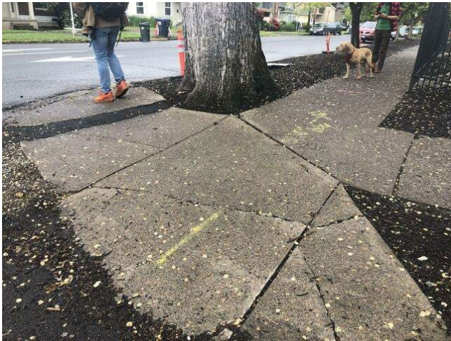
Figure 6. Sidewalk lacking curb cuts.
