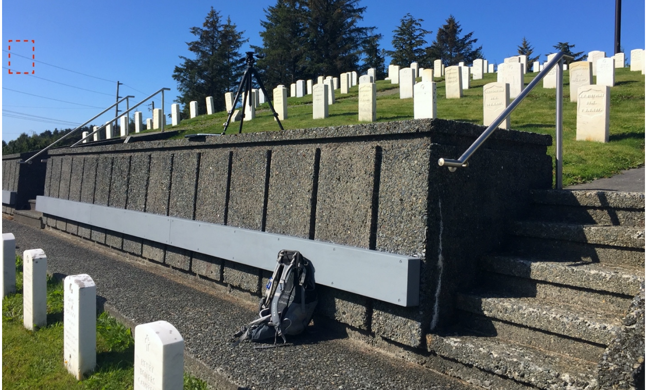
Figure 6-8. Post-WWII-era cut, retaining wall, and terrace below, view SE. The original camera station for S-05 was likely positioned on what is now a void. Calculated location of the actual point is approximated in box at upper left, while the tripod mount (visible at center-left) illustrates the would-be alignment of the view ahead of Merrill's lens.
