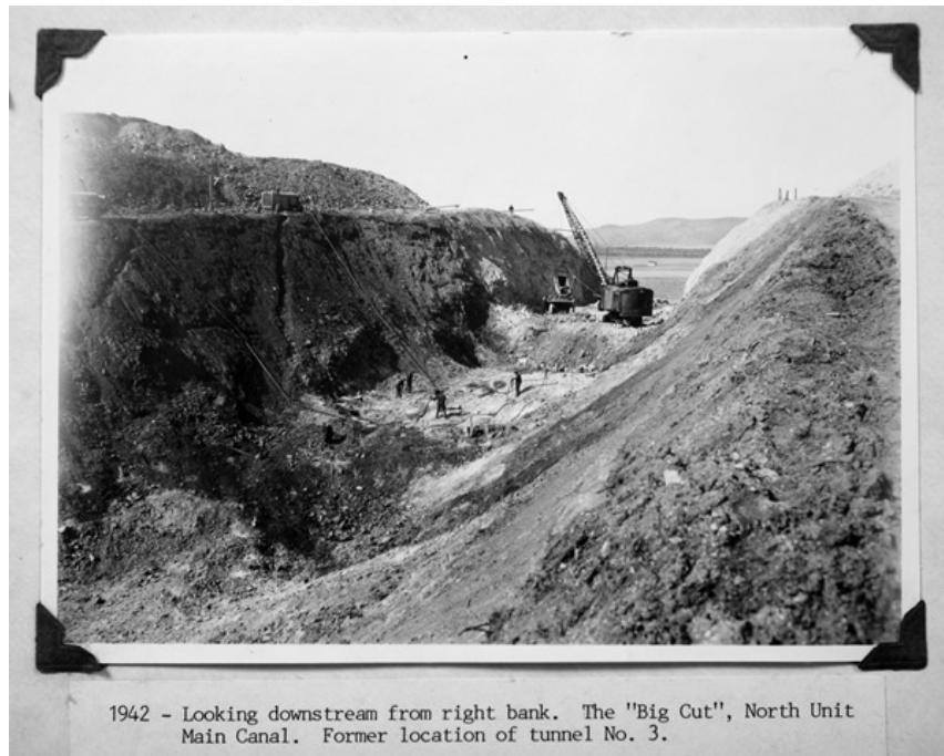
Figure 6. The ‘Big Cut’ – at least 40’ deep by its completion, allowed the Main Canal to connect to the waiting irrigation land just beyond the foothills of the Ochoco Mountains in the background. (North Unit Irrigation District, 2019).
