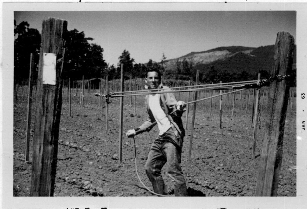
Figure 25 - Fastening the Wire to the Posts in a Pole Snap Bean Farm.
