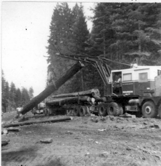
Fig. 38.--Loading Logs in the Woods. This is a heel-boom loader with a clam-shell grapple.
