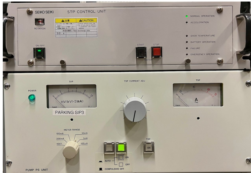
Figure 3.25. The turbo pump controls at the back of the room
