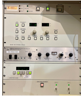
(b) The control panels for the MIED
