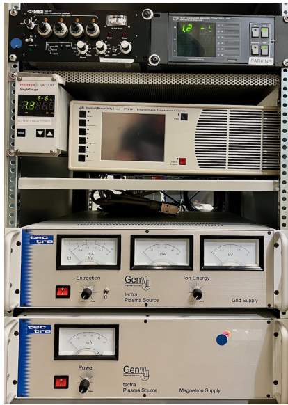
(a) The rack of controls for the plasma gun
